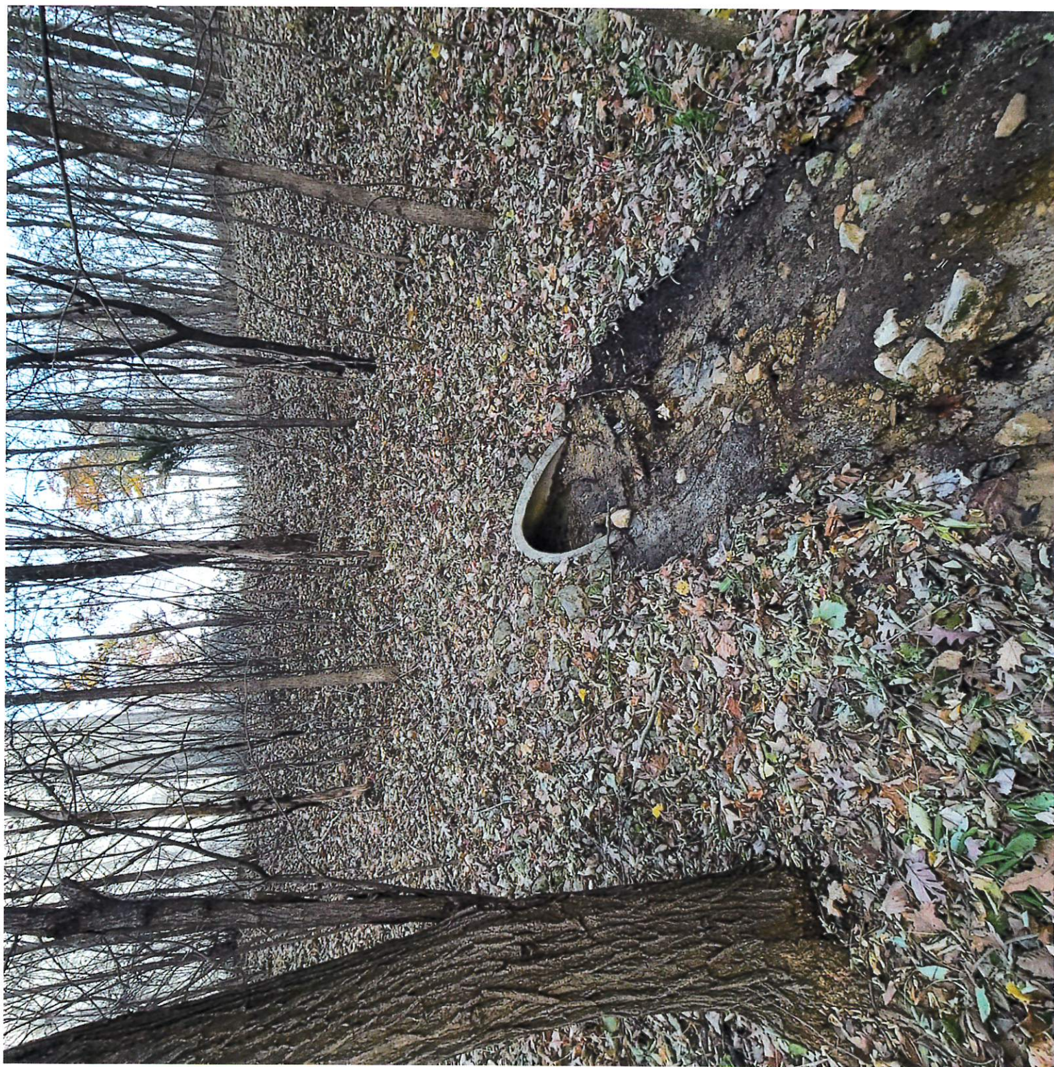
Reservoir PIP Discharge End
