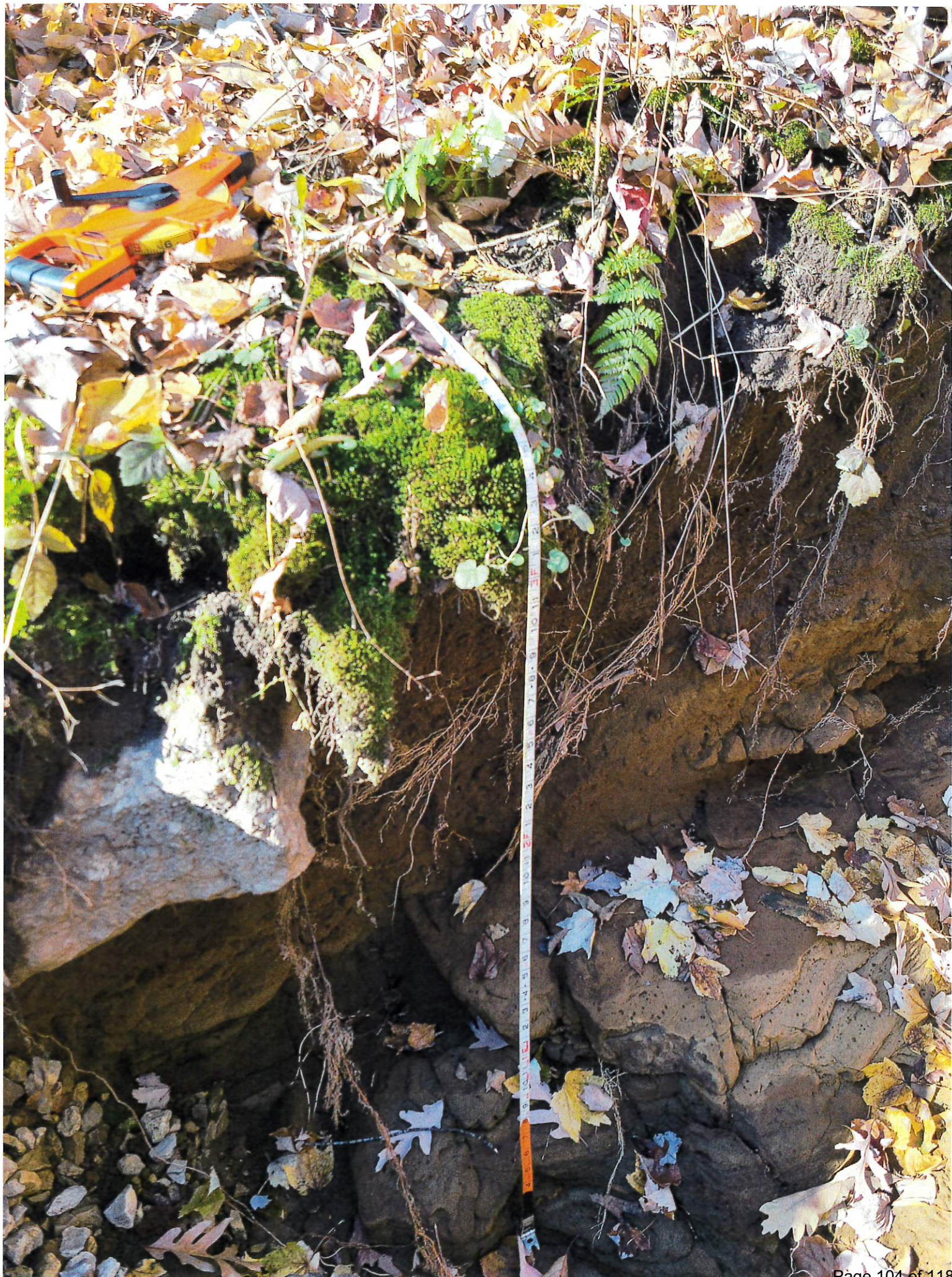
Depth @ a location in the eroded ditch
