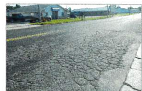
Existing severe pavement distresses near the Sauk County Facility Building.
