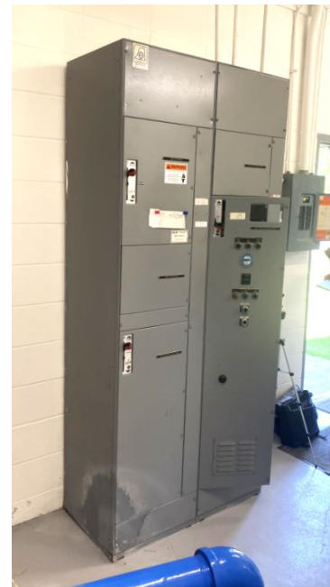
Existing Motor Control Center
