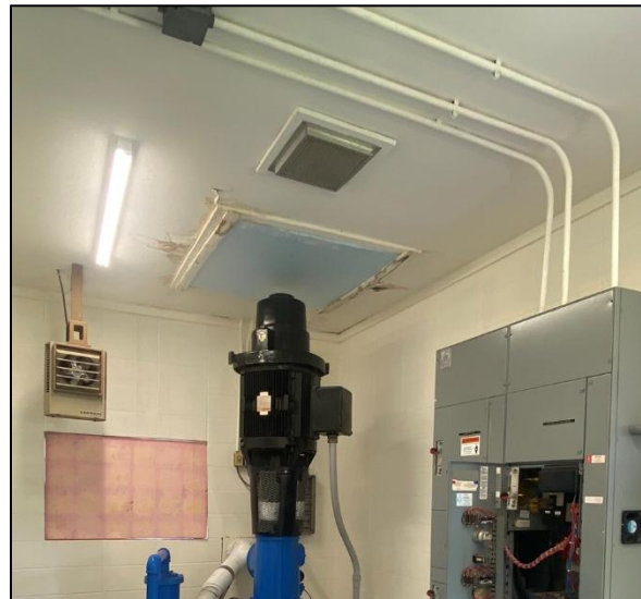
Roof Hatch Water Damage
