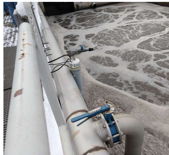
Air Distribution Piping & Valves
