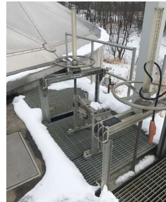
Flow Control Gates
