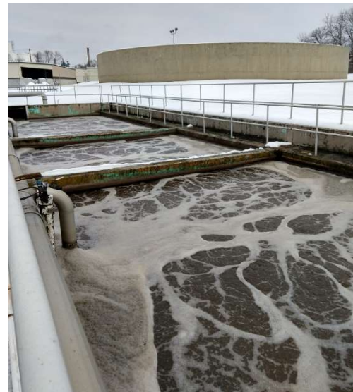
View of Aeration Basins from SW
