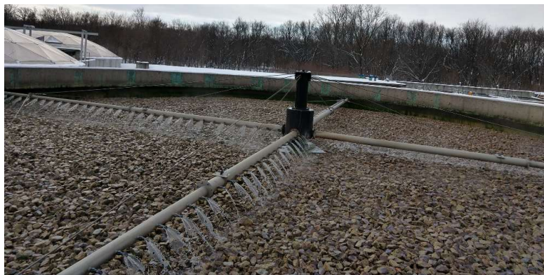
Top of Trickling Filter
