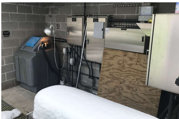
Effluent Auto-Sampler, Electrical Panels
