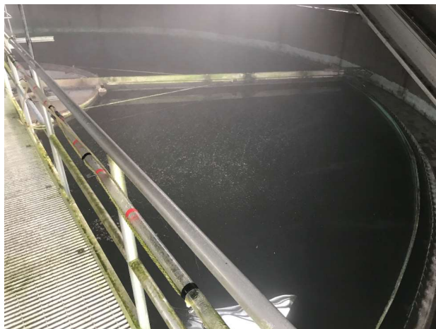
Final Clarifier Scum Rake, Launder, Walkway
