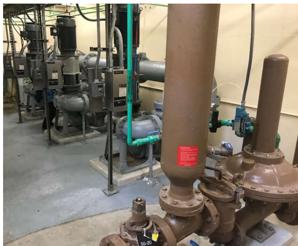
Pumps in Basement
