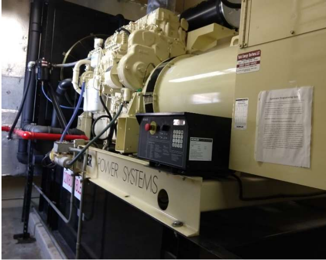
Standby Diesel Generator
