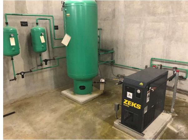
Air Receiving Tank and Drier
