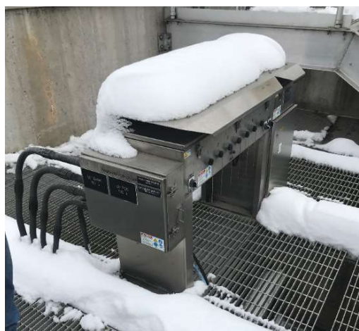
UV Disinfection System
