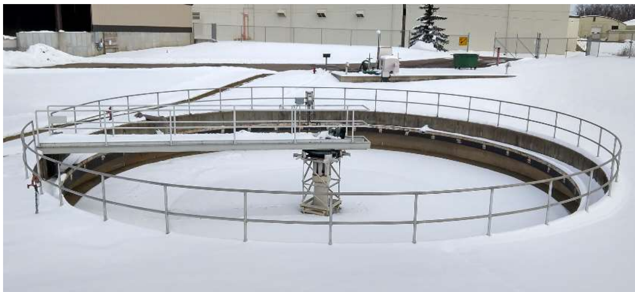
Top of Centrate Holding Tank
