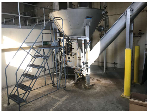
Side of Vulcan Grit Washing System
