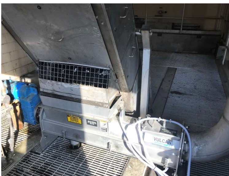
Back of Vulcan Step Screen & Washer/Compactor
