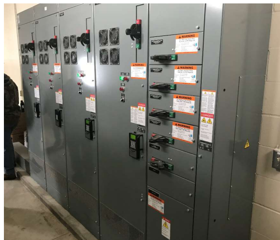
Motor Control Center in Electrical Room
