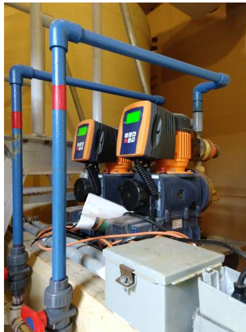
Chemical Feed Pumps
