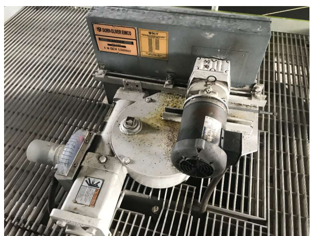
Final Clarifier Drive
