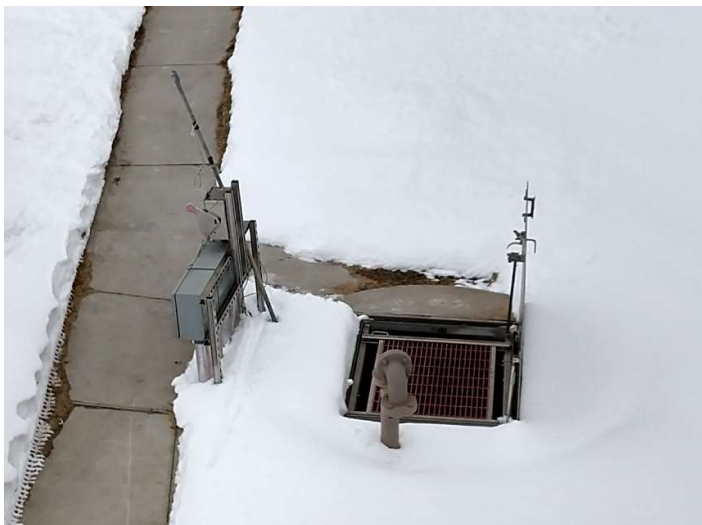
Side View of Centrate Pump Station
