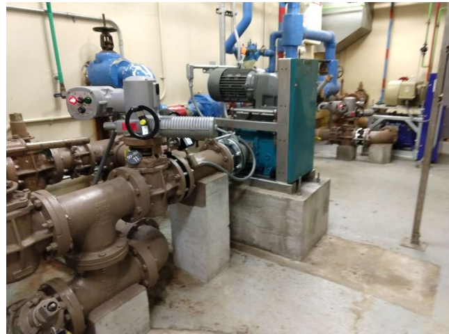
Additional Pumps in Basement
