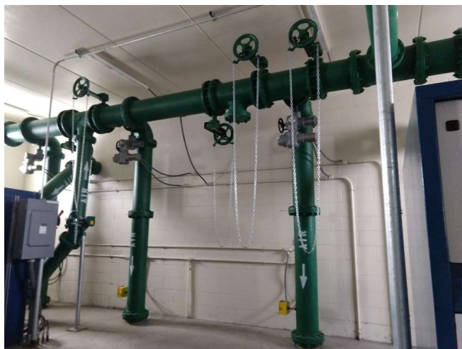
Air Piping Within New Blower Building
