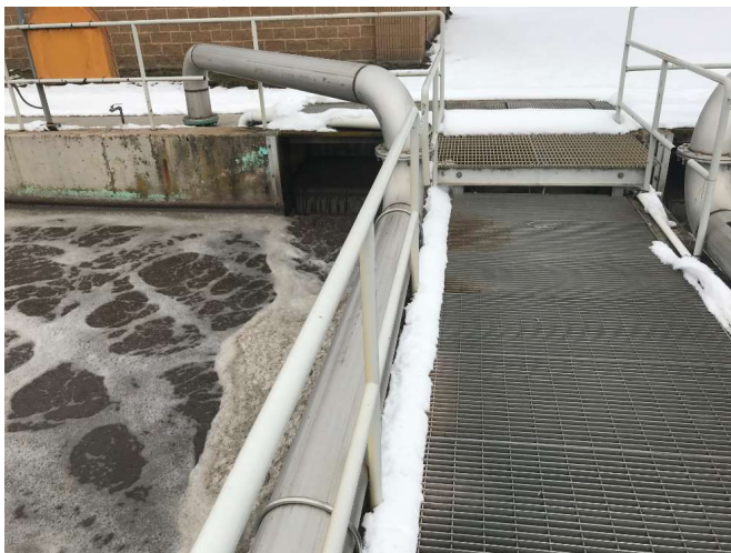
Air Distribution Piping & Walkway
