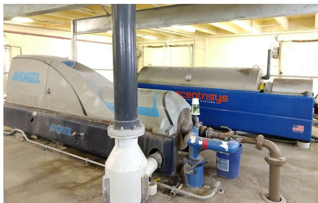
Sludge Dewatering Centrifuges
