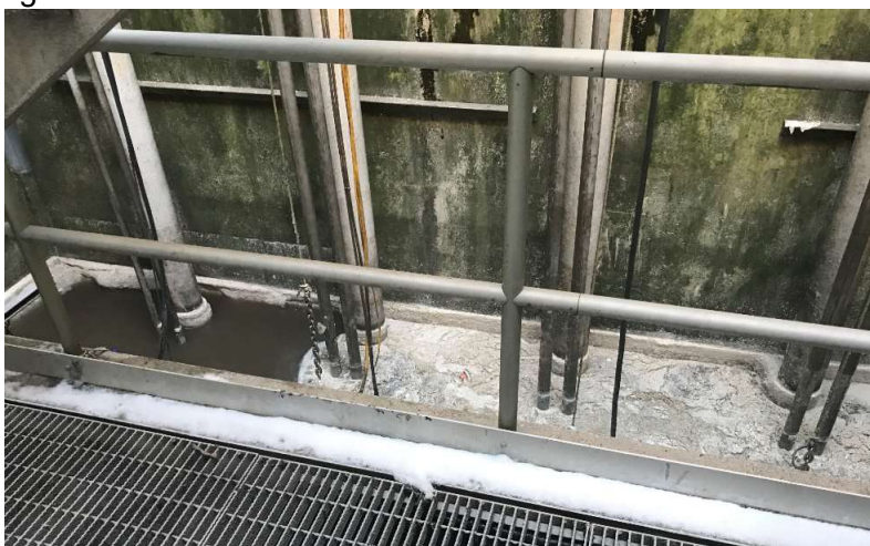
Submersible Raw Sewage Pumps
