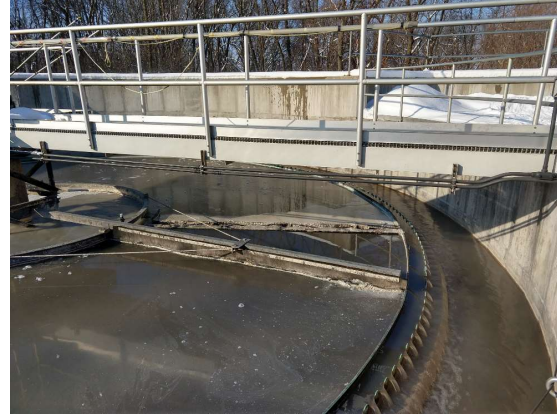
Interior of Circular Primary Clarifier
