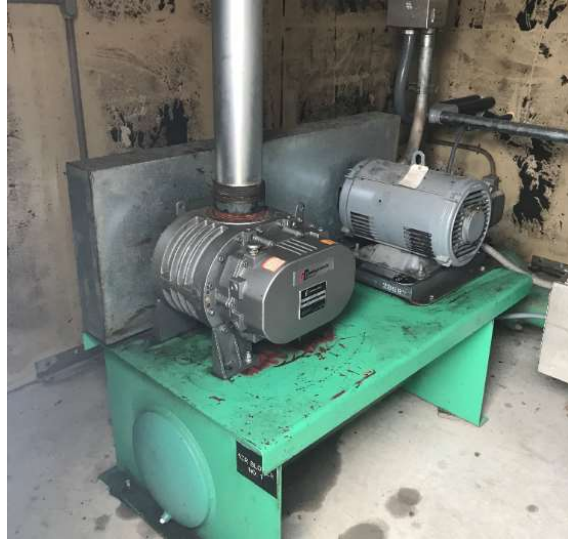
Blowers Inside Blower Shed
