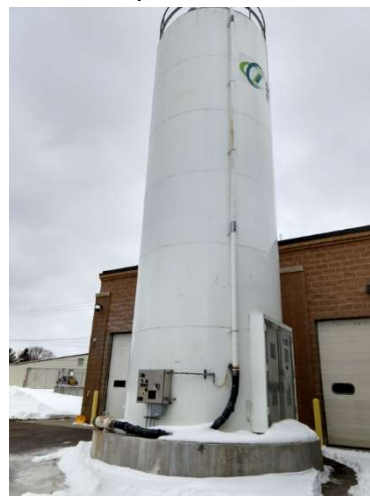
Lime Storage Silo
