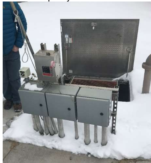
Front View of Centrate Pump Station
