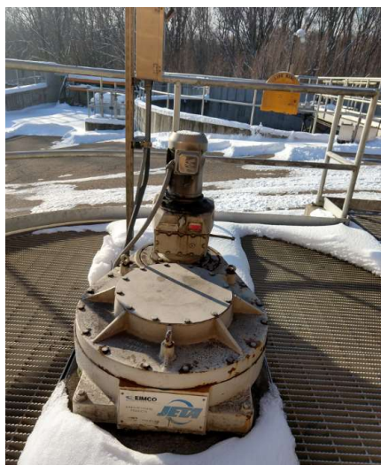
Grit Removal System
