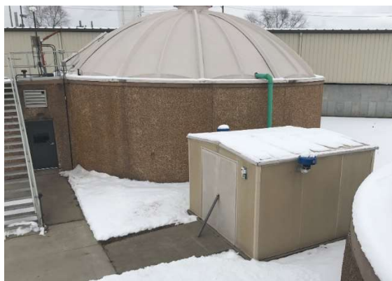
North Holding Tank & Blower Shed
