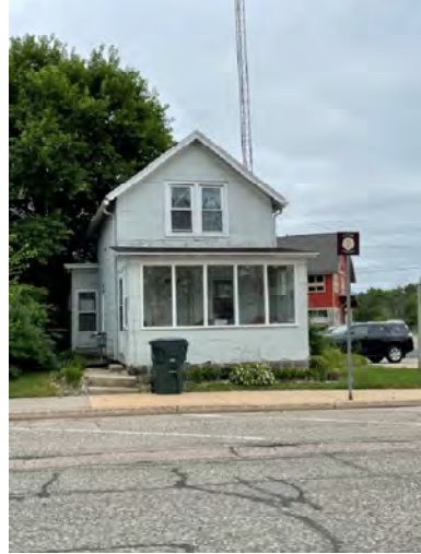
MAP ID 20 - Parcel 1006: 136 Vine Street. Deteriorating structure and site improvements
