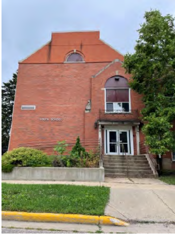
MAP ID 50 - Parcel 1640: 420 Plum Street. Deteriorating structure.
