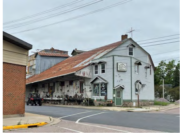
MAP ID 41 - Parcel 1054: 310 Railroad Street. Deteriorating roof and structure. Age of building. Deteriorating site improvements.
