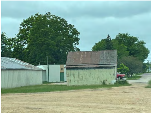
MAP ID 54 - Parcel 480: 430 South Avenue. Deteriorating building. Old and obsolete. Parcel does not meet standards.
