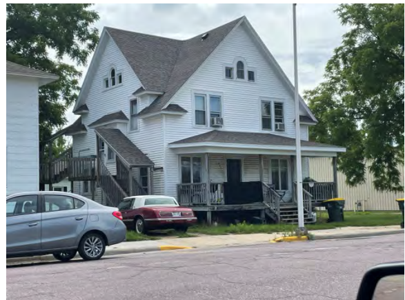
MAP ID 38 - Parcel 1035: 247 S. Park Street. Deteriorating deck and site improvements.
