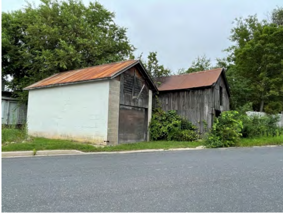
MAP ID 18 - Parcel 1005: Rear of lot – deteriorating site improvements.
