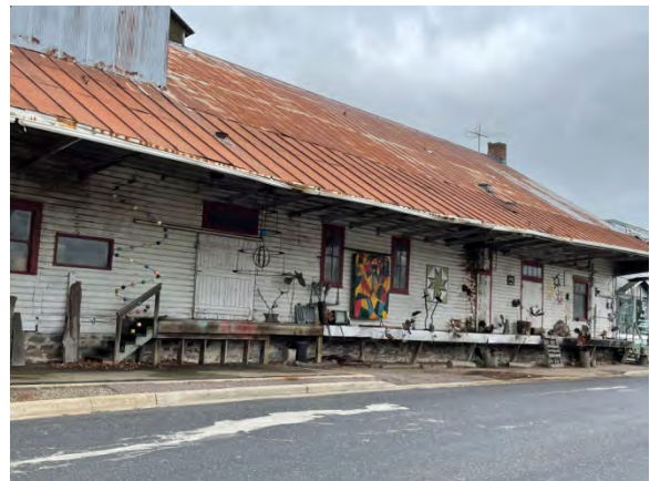
MAP ID 41 - Parcel 1054: See above. Old and deteriorating structure and site improvements.
