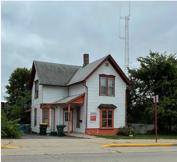
MAP ID 31 - Parcel 958: 340 E. Main Street. Deteriorating site improvements and structure. Age of property.
