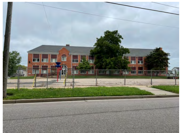
MAP ID 50 - Parcel 1640: 420 Plum Street. Deteriorating site improvements.
