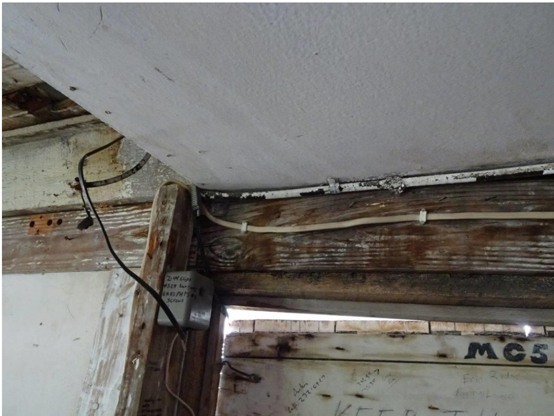
Photo 4.2.22 – Exposed Outdated Electrical Wiring
