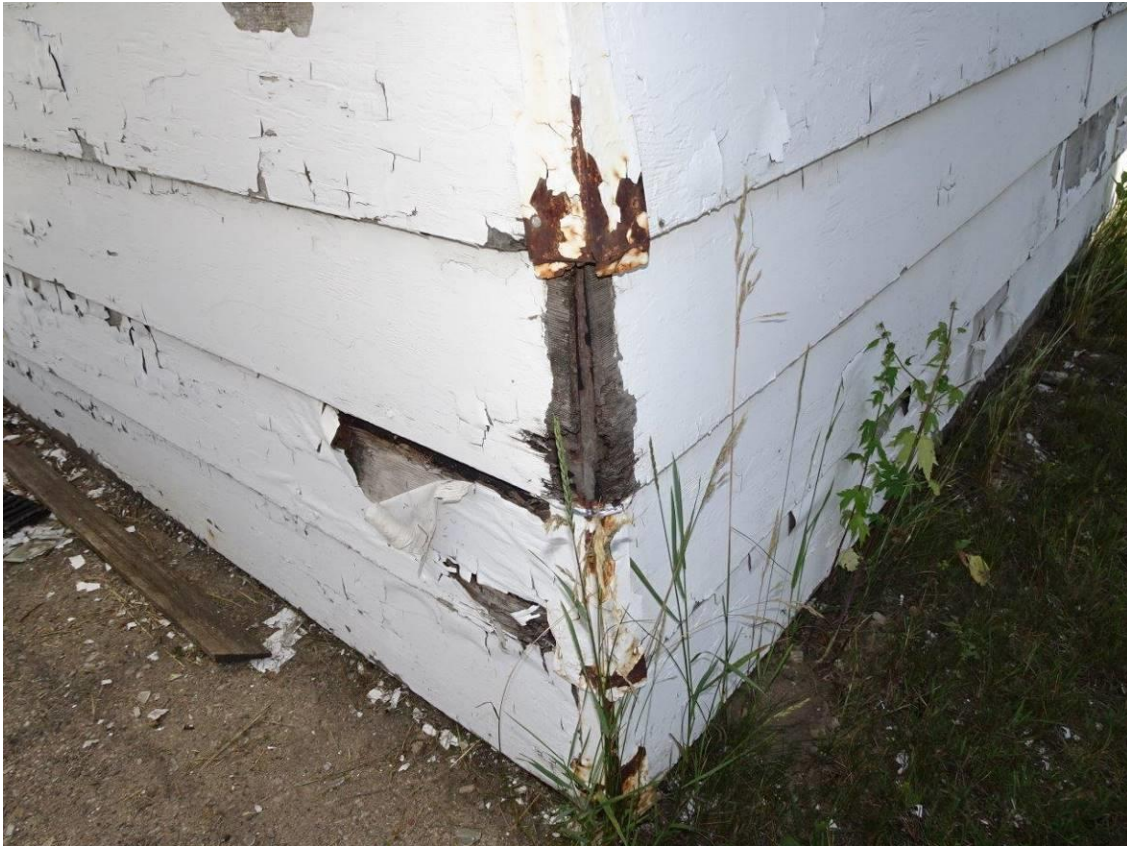
Photo 4.1.15 – Neglected Paint and Maintenance at Building Siding and Trim
