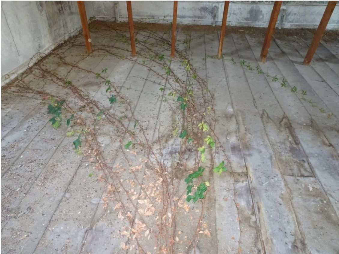
Photo 4.2.13 – Vines Growing into the Building and Across the Attic / Loft Floor
