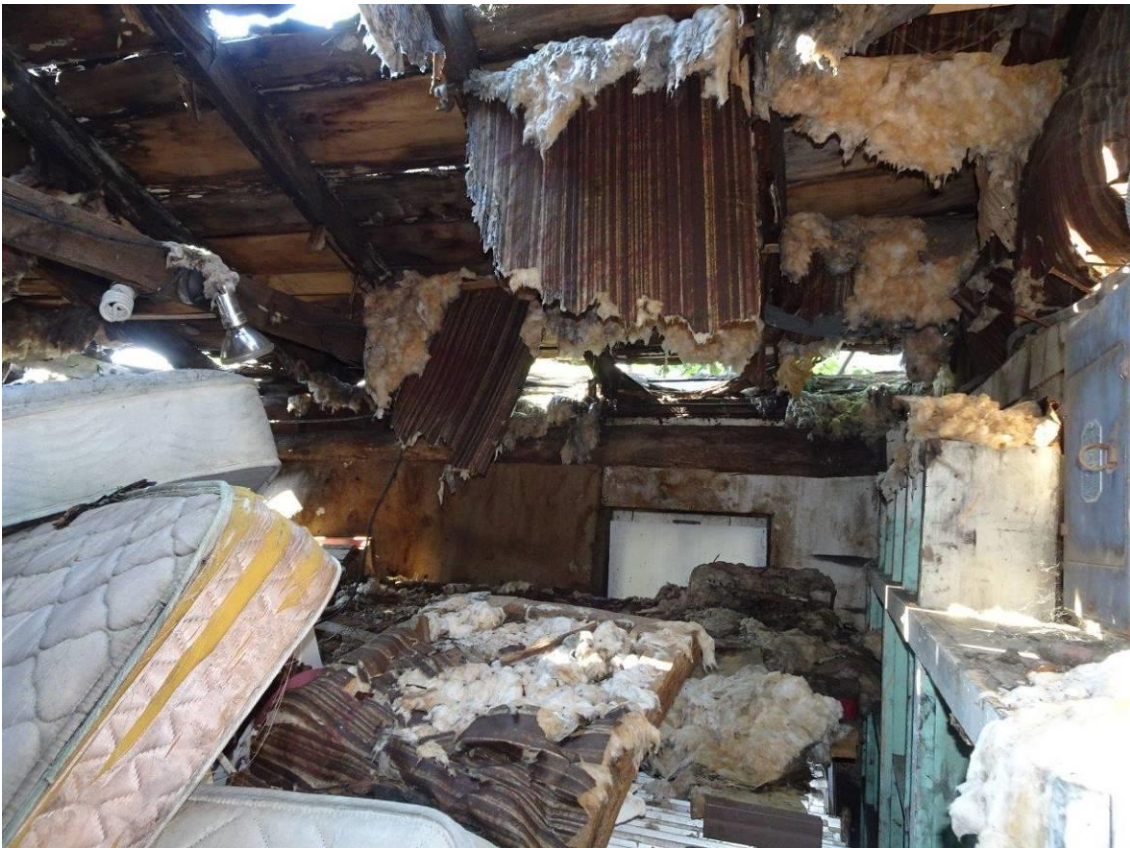
Photo 4.3.7 – Hanging Weathered and Water Sodden Roof and Wall Insulation
