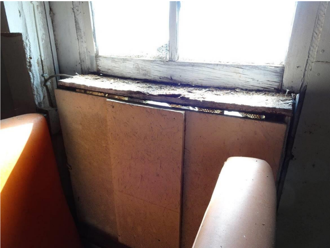
4.2.16 – Rotting Sills and Walls Inside Dilapidated Openings
