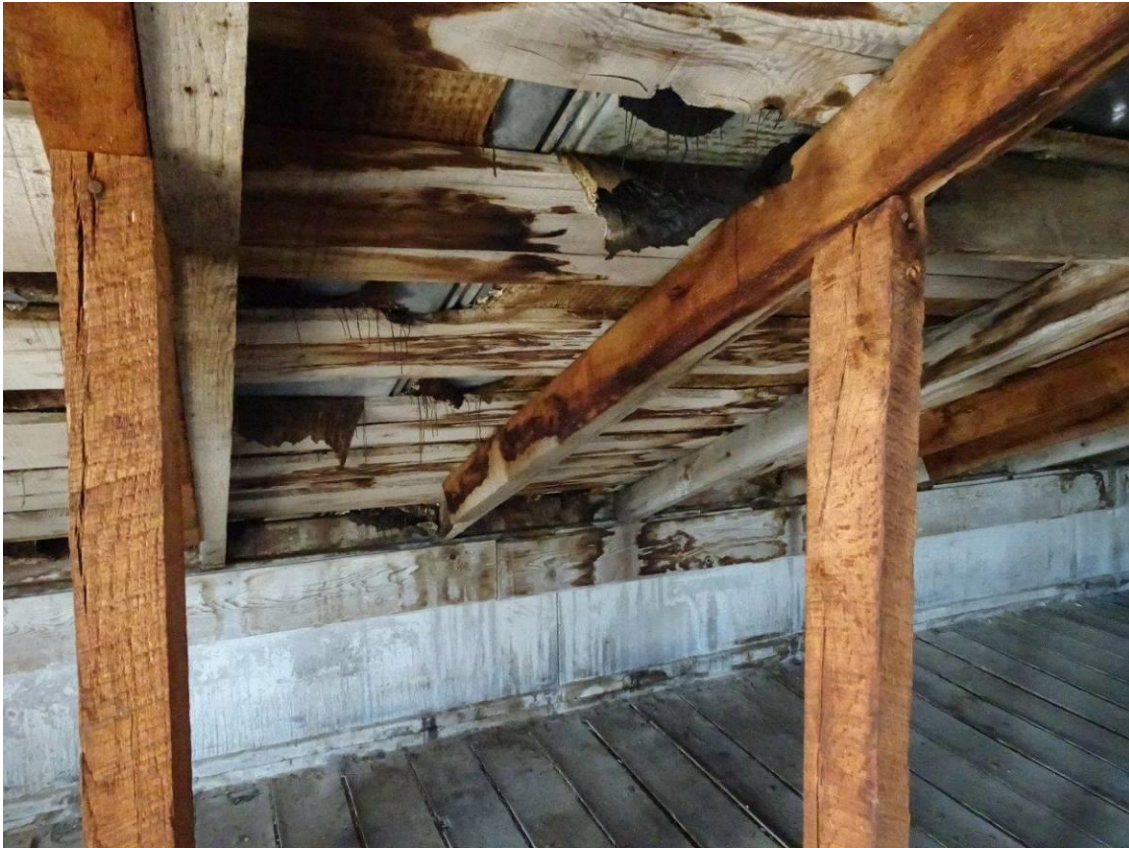
Photo 4.2.19 – Rotting Roof Rafters and Wood Board Sheathing – No Roof Insulation
