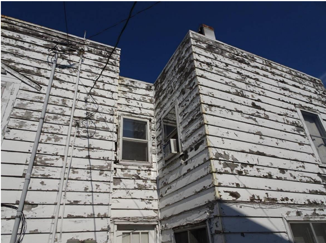
Photo 4.1.10 – Dilapidated Exterior Siding and Trim Paint – Maintenance Neglect
