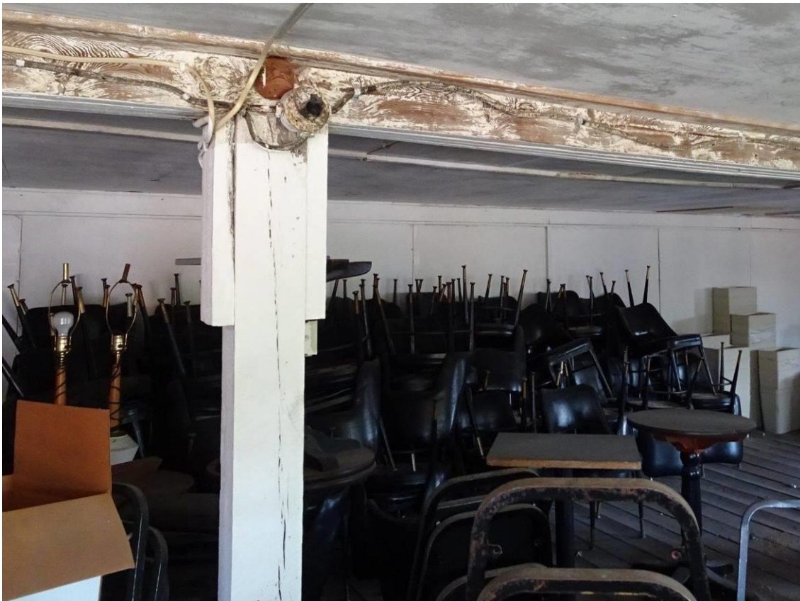
Photo 4.2.28 – Congested Storage, Exposed Outdated Wiring and Broken Light Fixtures
