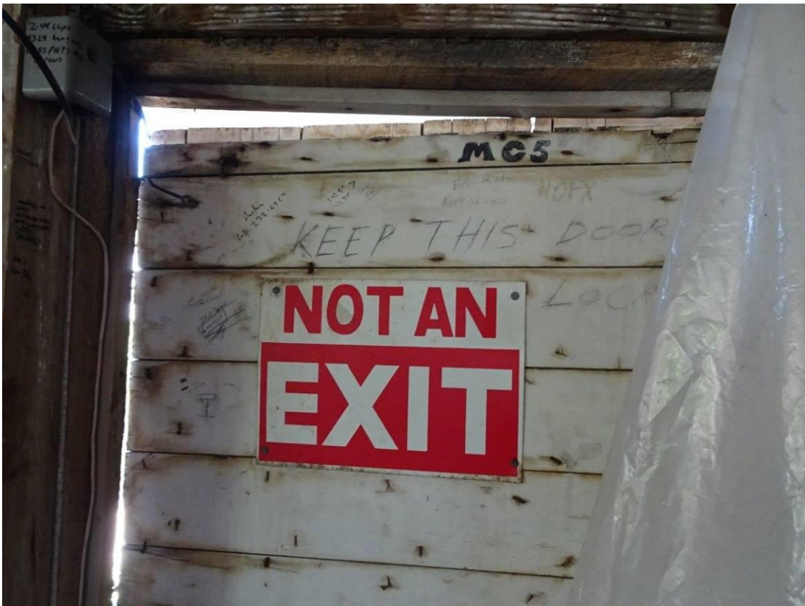
Photo 4.2.26 – Unprotected Outswing Second Floor Door with No Landing Outside and Hook Latch Interior
