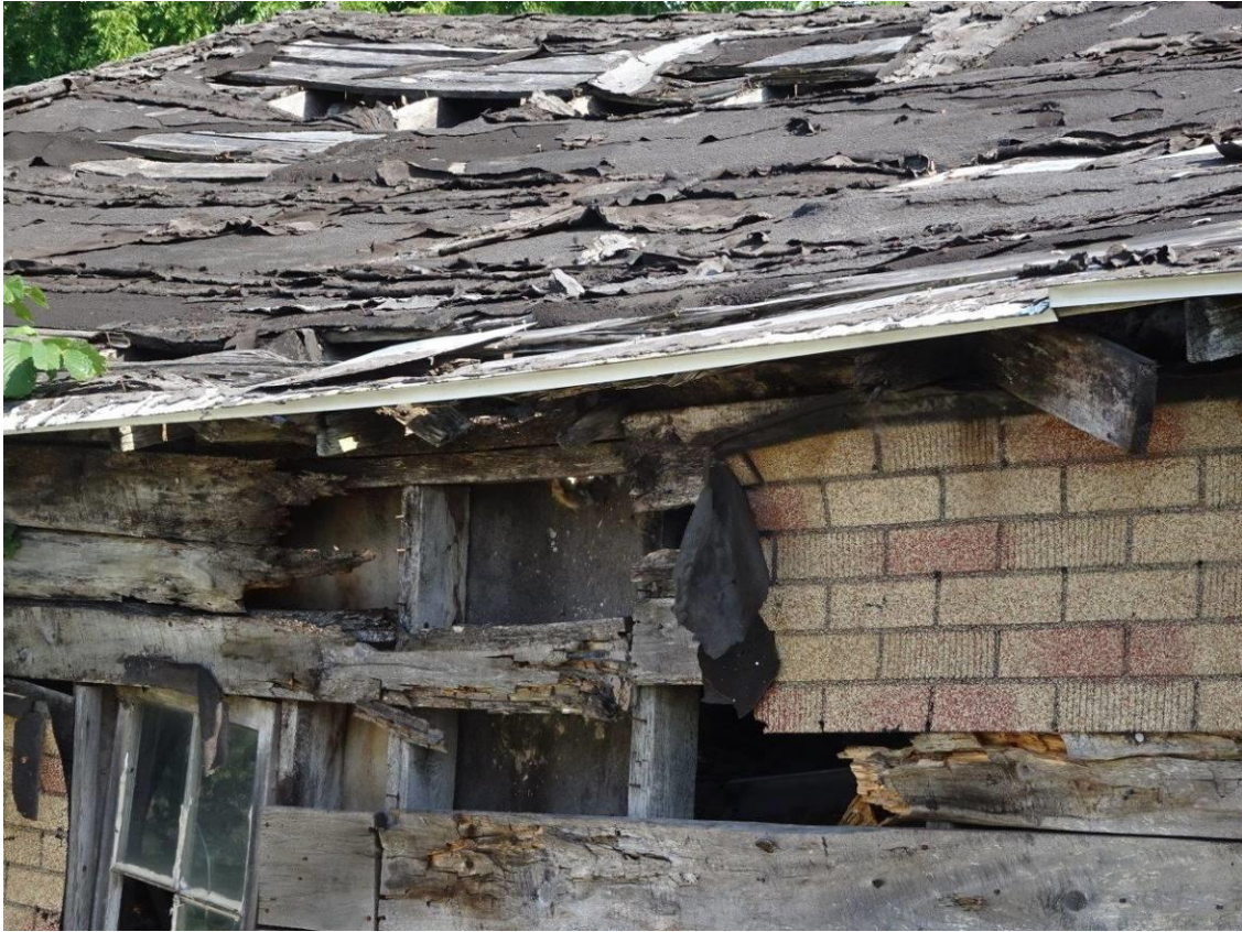
Photo 4.3.10 – Rotting and Collapsing Exterior Walls and Roof
