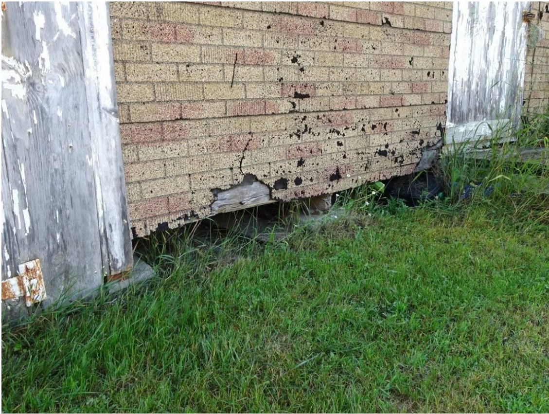
Photo 4.3.4 – Wood Posts Bearing On Concrete Pads at Grade – Rotting Base of Walls
