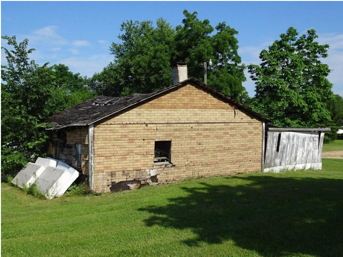
Photo 4.3.1 – Dilapidated Storage Shed
