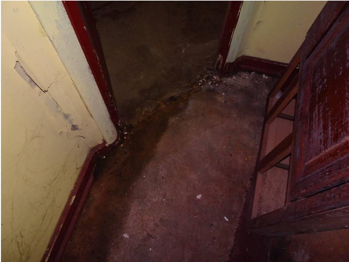
Photo 4.1.17 – Damp Floors from Wall and Door Leaks
