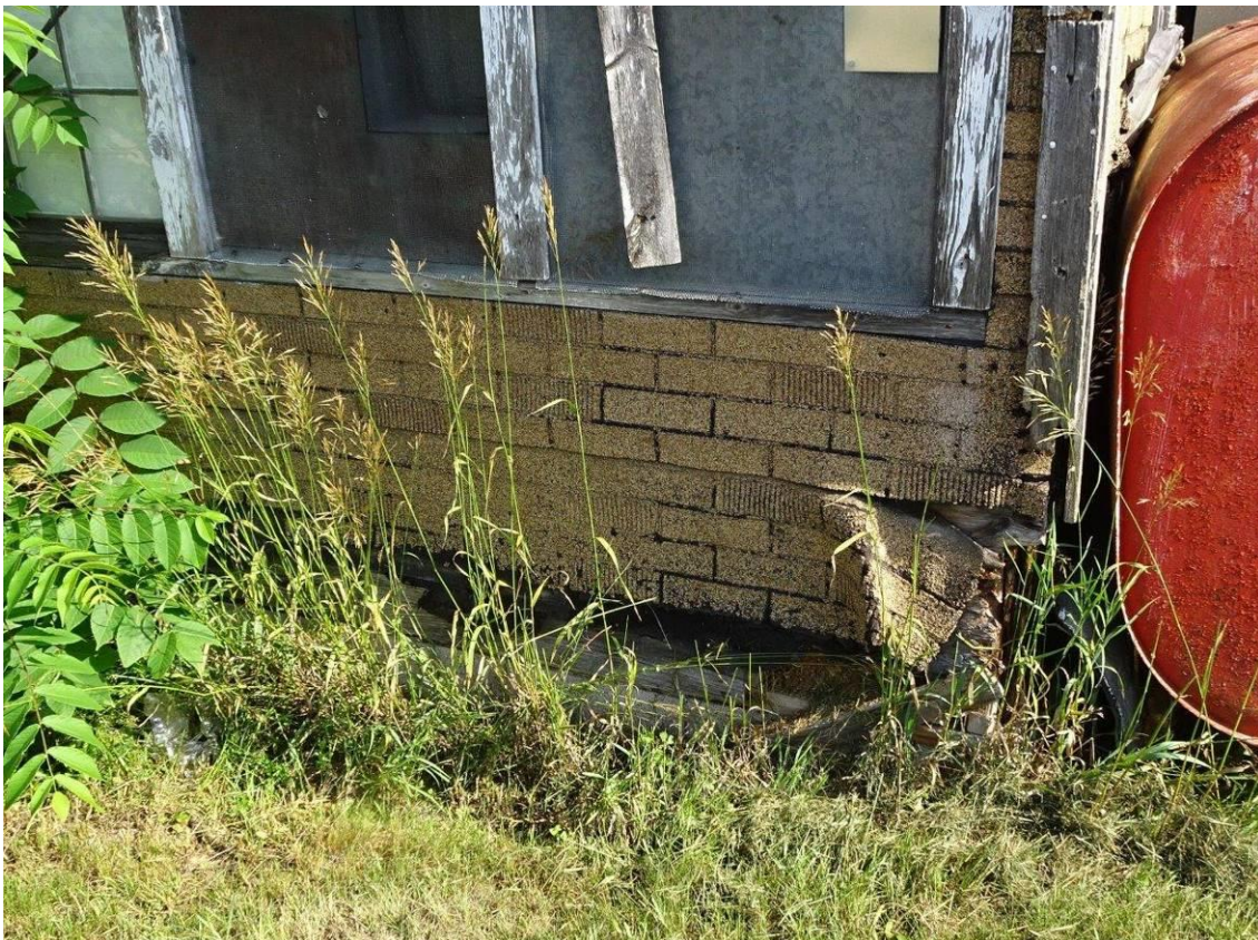
Photo 4.2.12 – Rot at Base of Walls from Water Infiltration
