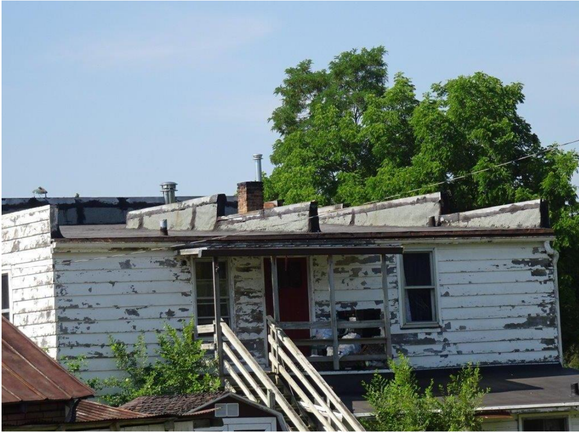
Photo 4.1.28 – Questionable Roof Finish Integrity
