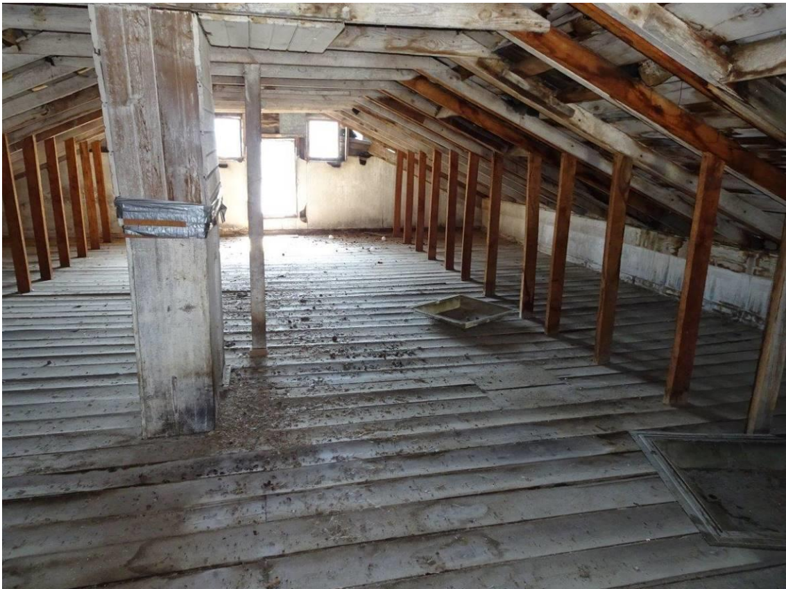
Photo 4.2.18 – Attic Framing with Supports and Sleepers Added – Water Damage to Framing & Floors
