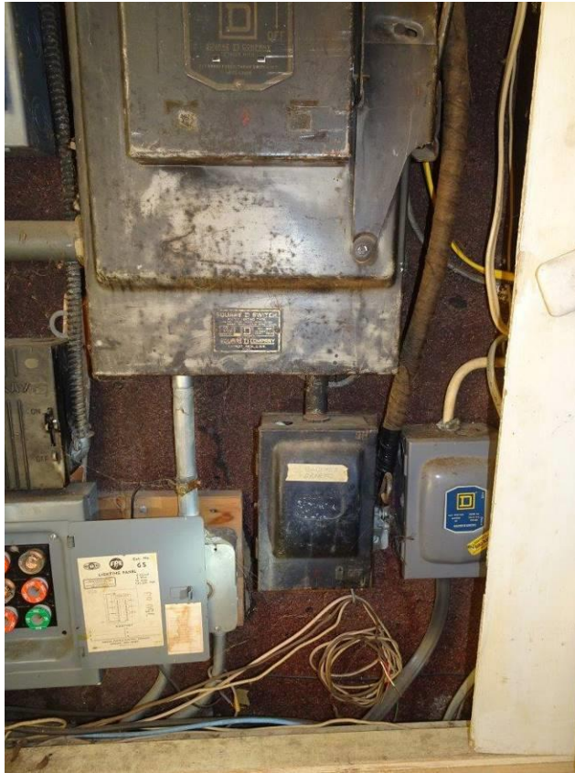
Photo 4.1.19 – Outdated Electrical Service Panels
