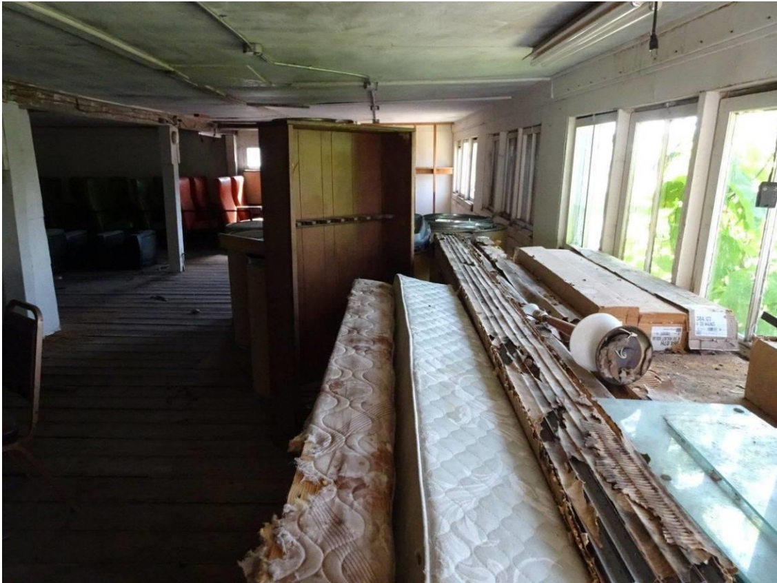
Photo 4.2.29 – Rotting Mattresses Stacked Against Broken and Missing Window Openings
