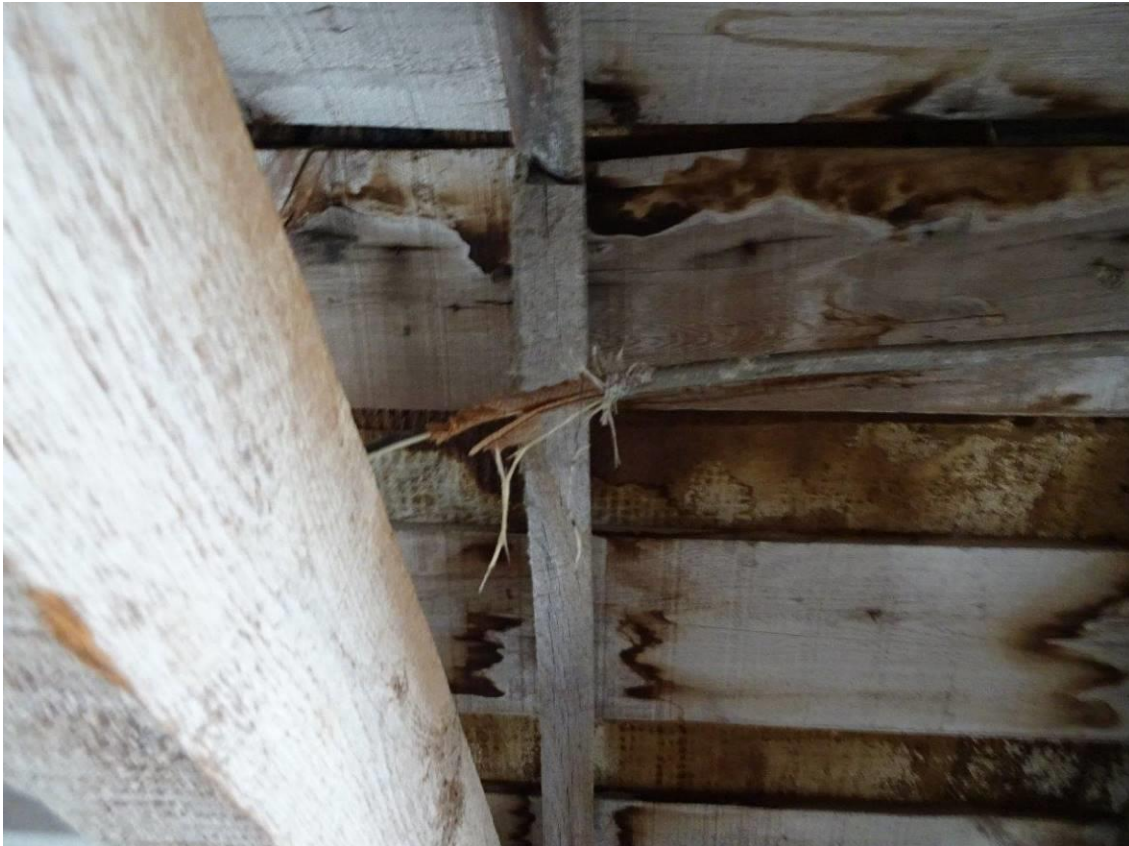
Photo 4.2.31 – Exposed Outdated Wiring with Bare Wires in Contact with Wood Framing
