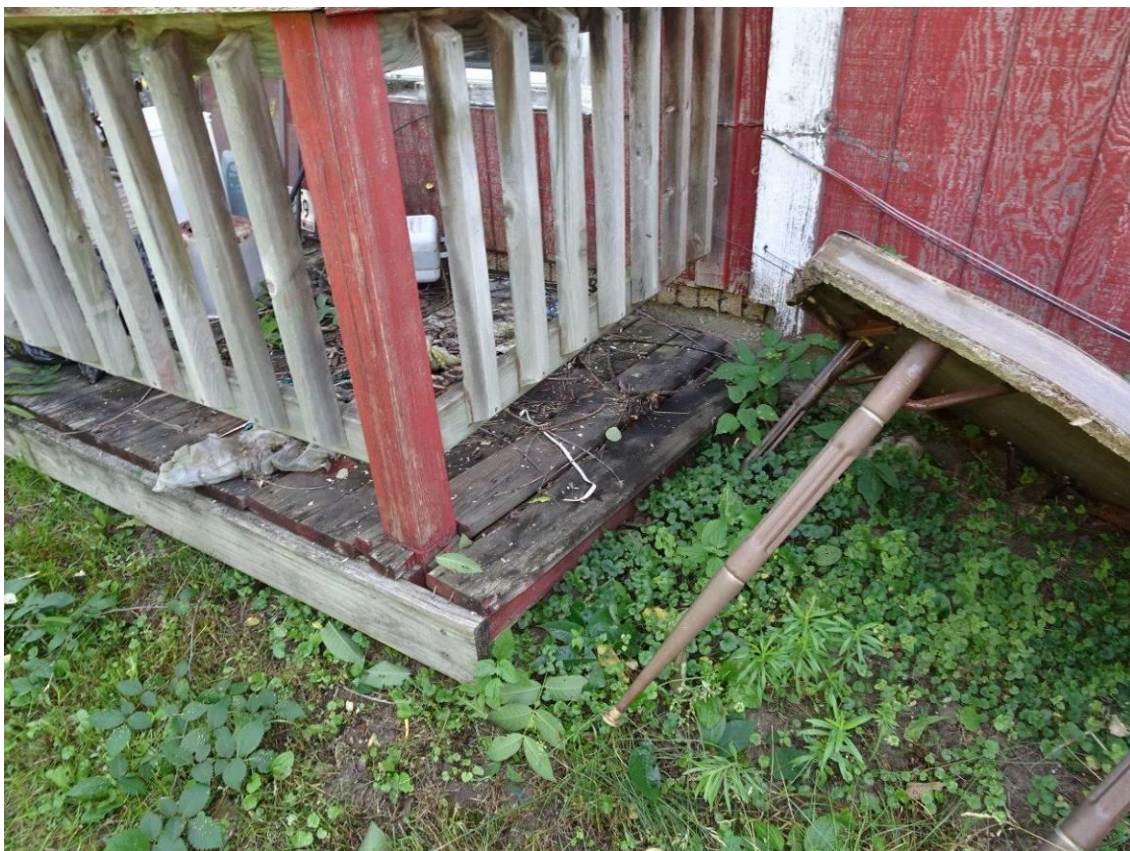
Photo 4.1.27 – Dilapidated Wood Deck Rotting Away From Building
