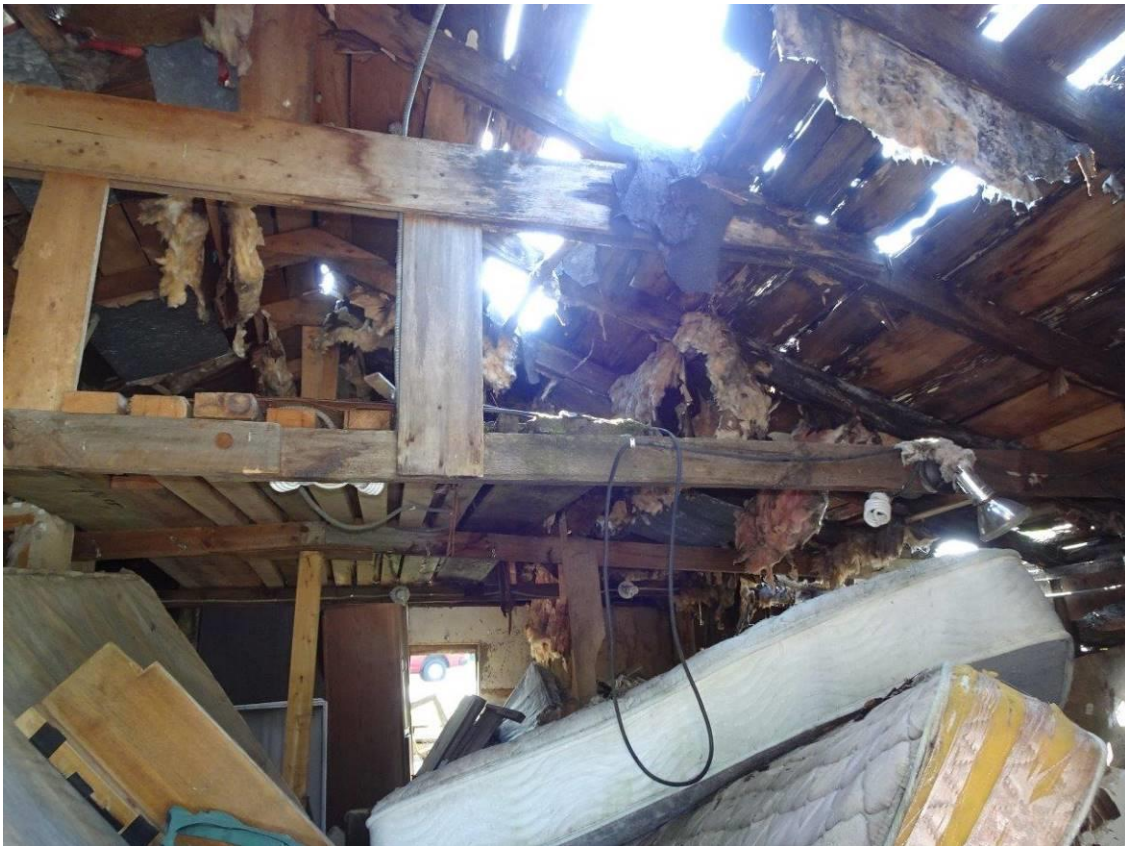
Photo 4.3.8 – Rotting Roof Framing and Sheathing with Numerous Large Holes Fully Exposed to Weather
