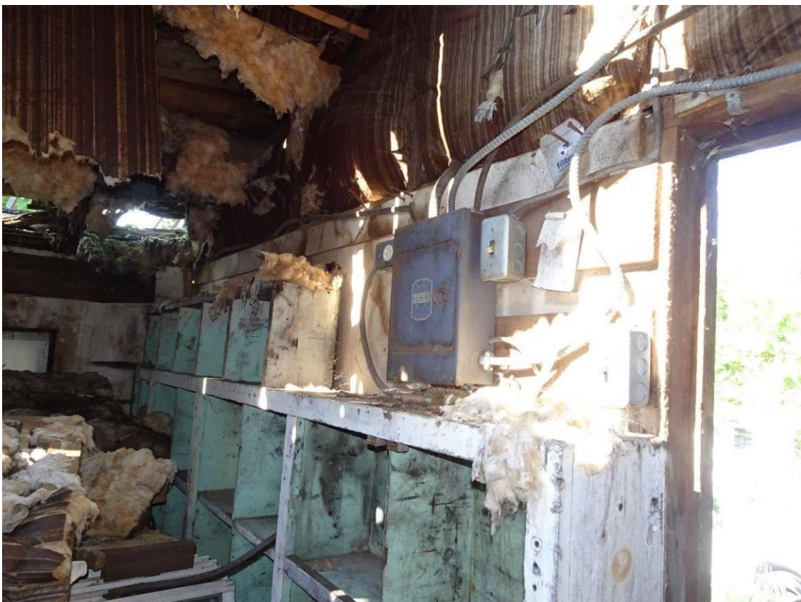
Photo 4.3.9 – Exposed Electrical Panels and Wiring Beneath Open Sky Rotting Roof Openings
