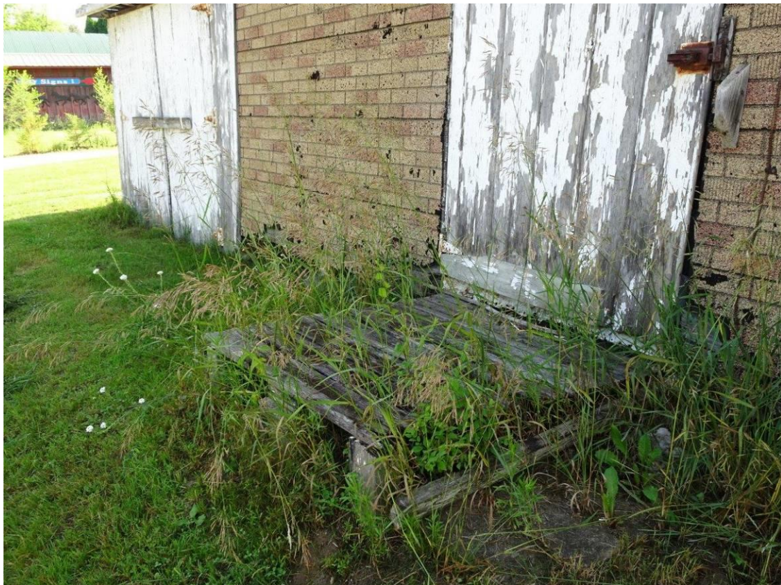
Photo 4.3.13 – Rotting Wood Door Stoop with Missing Board Sections
