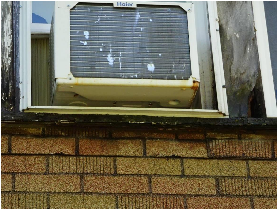
Photo 4.1.13 – Rotting Wall and Finishes Due to Degraded Window Flashing and Sealants
