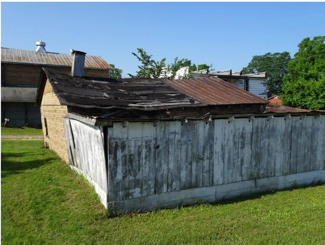
Photo 4.3.3 – North Lean-To Addition with Completely Collapsed Roof and Leaning Walls
