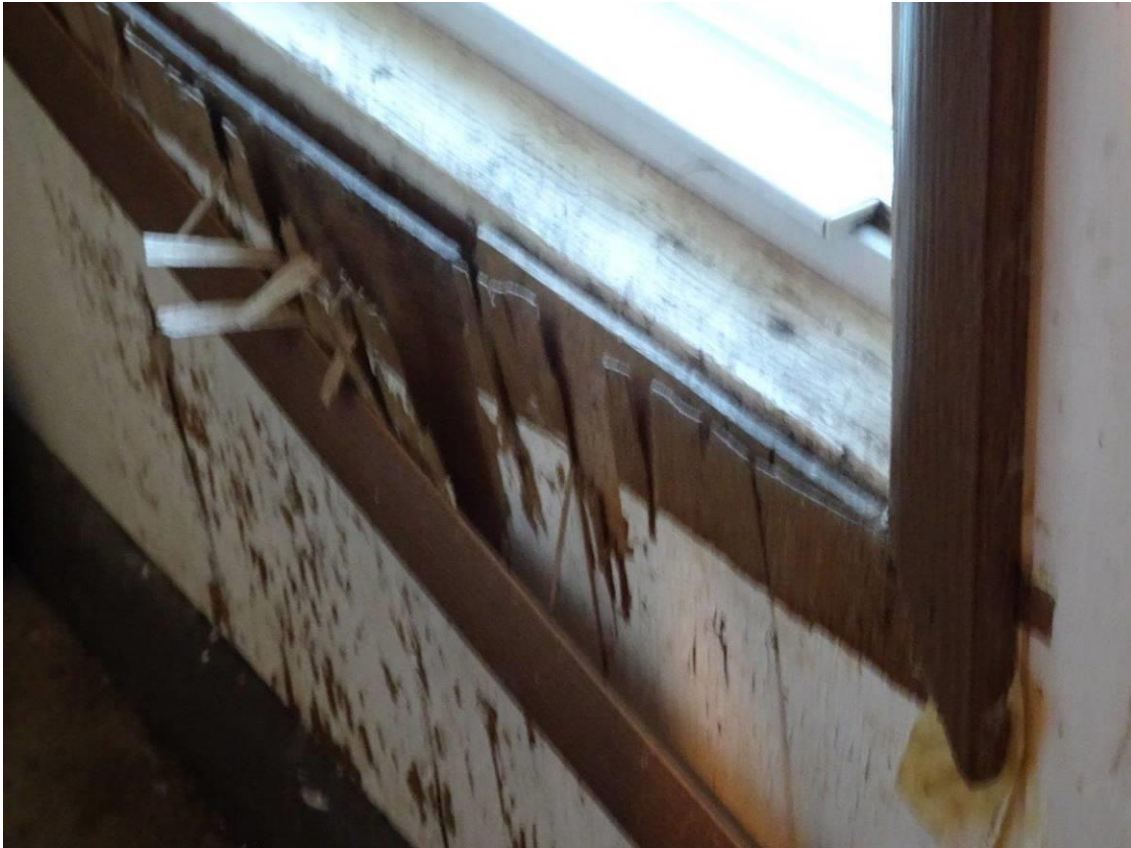
Photo 4.1.9 – Wall Finish and Trim Rotting at Window Leaks
