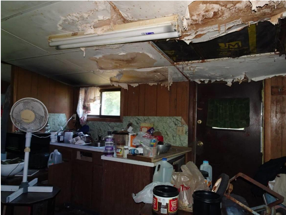
Photo 4.1.24 – Falling Ceiling from Ceiling Leak and Rusting Ceiling Grid
