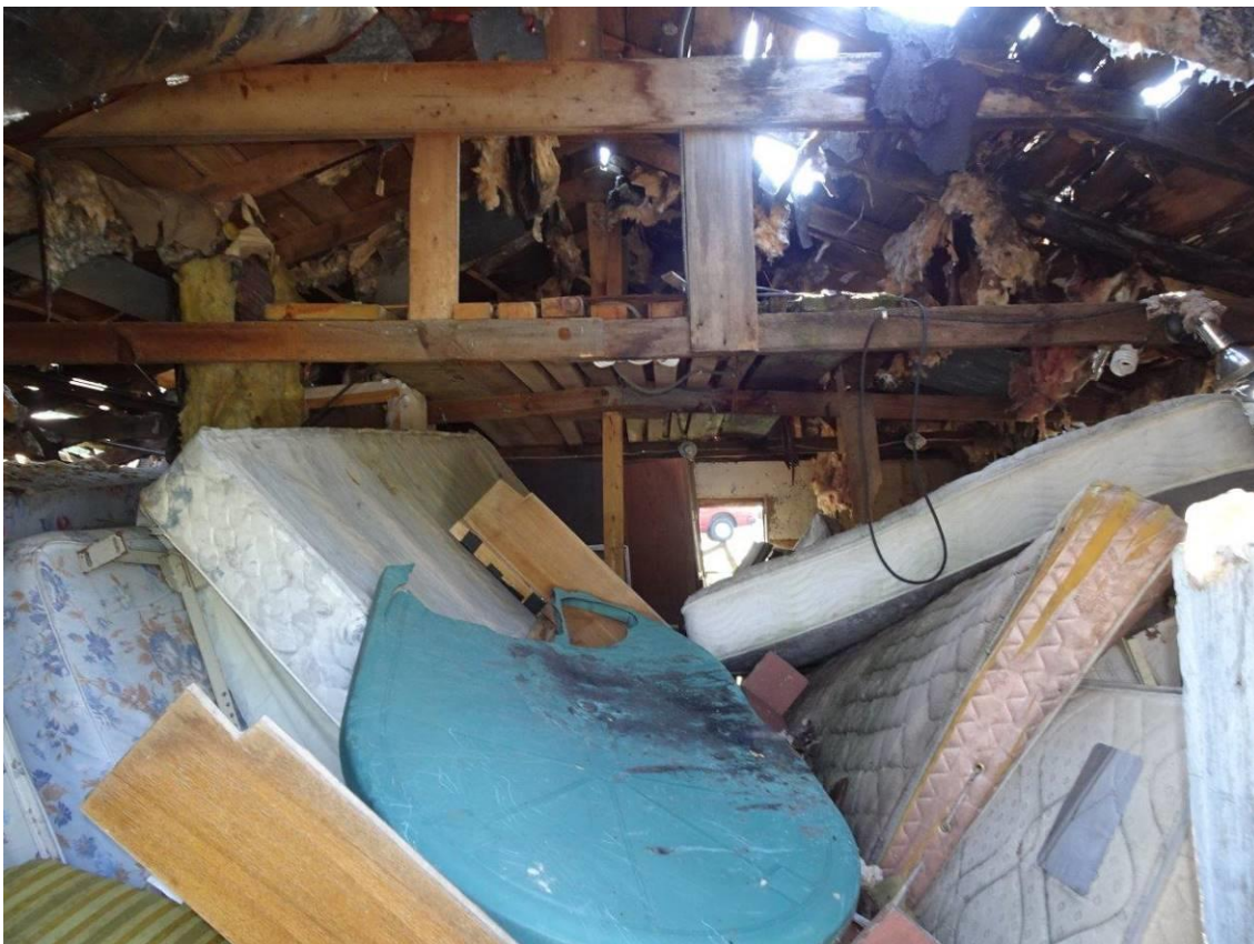
Photo 4.3.5 – Rotting Stored Mattresses Filling Interior Posing Mold and Fire Hazard
