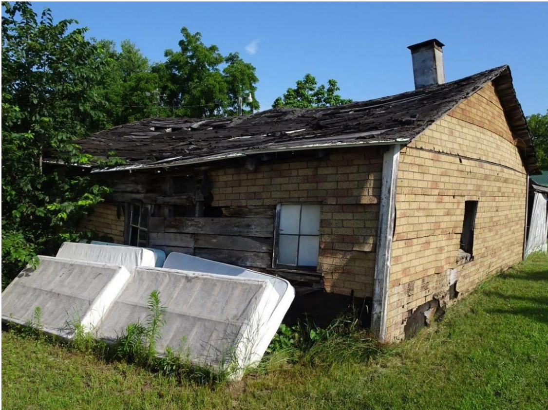
Photo 4.3.12 – Rotting Flammable Storage Both Interior and Exterior – Falling Decommissioned Chimney
