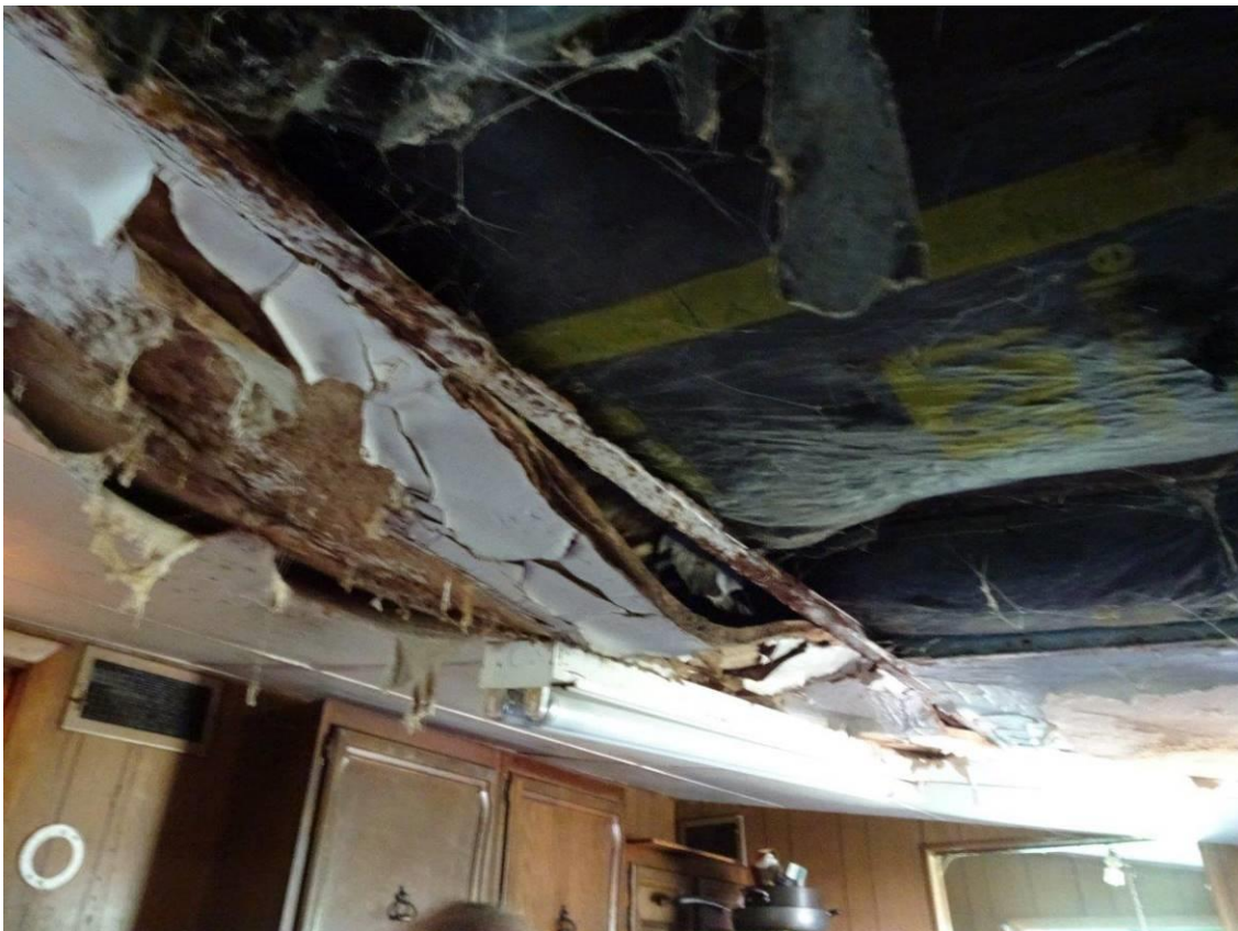
Photo 4.1.25 – Falling Ceiling and Insulation Pulling Light Fixtures Down with Ceiling
