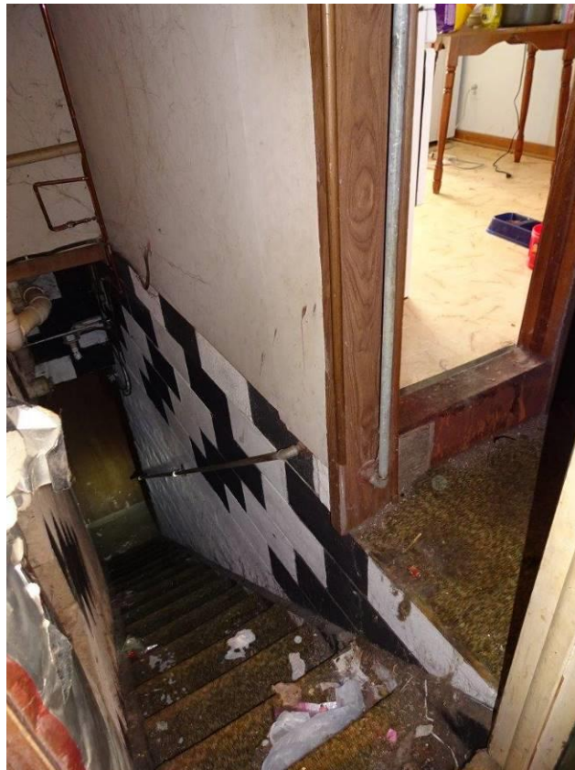
Photo 4.1.29 – Dangerous Non-Code Compliant Kitchen Entry Door Off Stair Side
