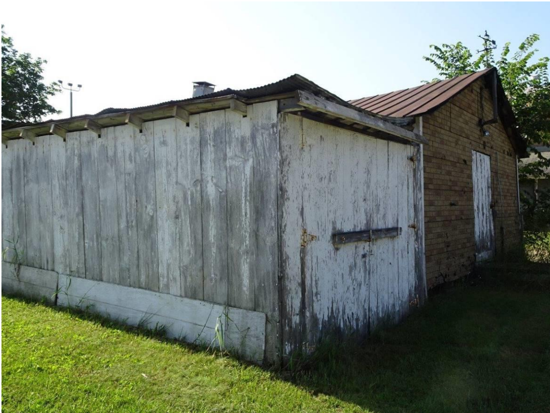
Photo 4.3.2 – North Lean-To Addition with Rotting, Unsecured Doors
