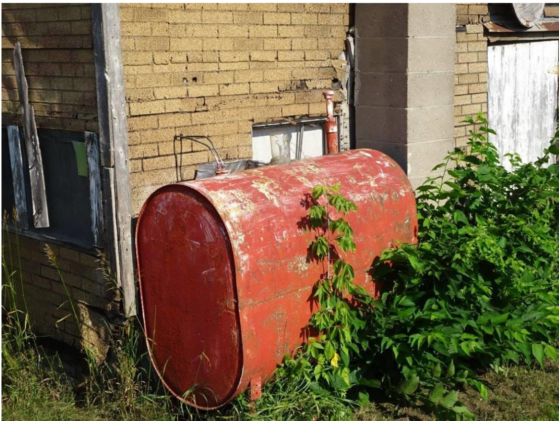
Photo 4.2.20 – Rusting Decommissioned Waste Oil Tank
