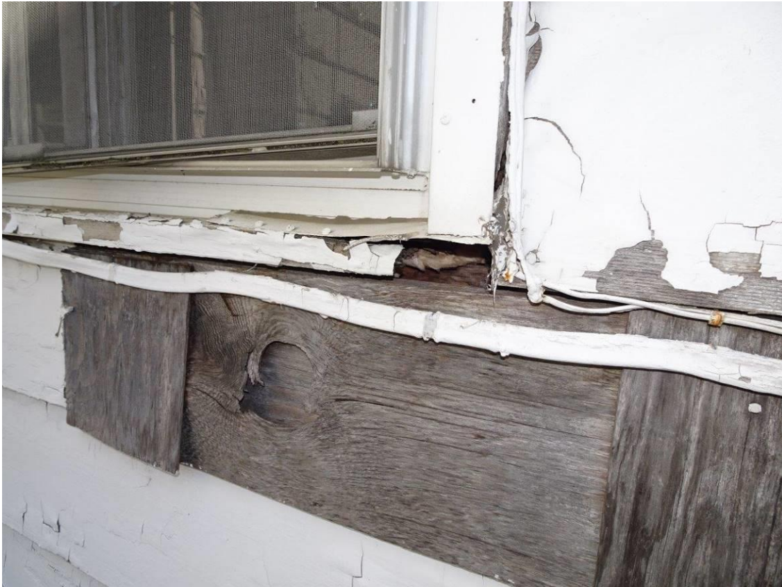
Photo 4.1.11 – Wall Cavities Exposed at Dilapidated and Missing Flashing and Sealants
