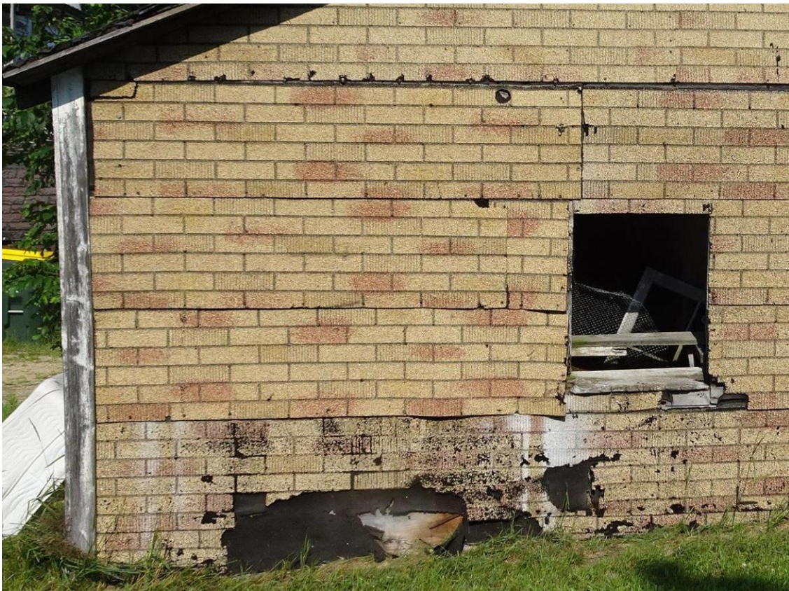
Photo 4.3.11 – Unsecured Building with Missing Windows – Rotting Wall Framing
