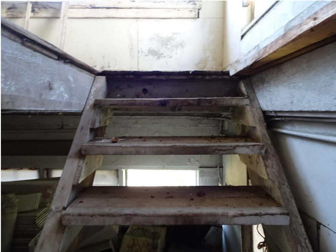
Photo 4.2.25 – Unprotected Stair Openings with No Guardrails and No Handrails
