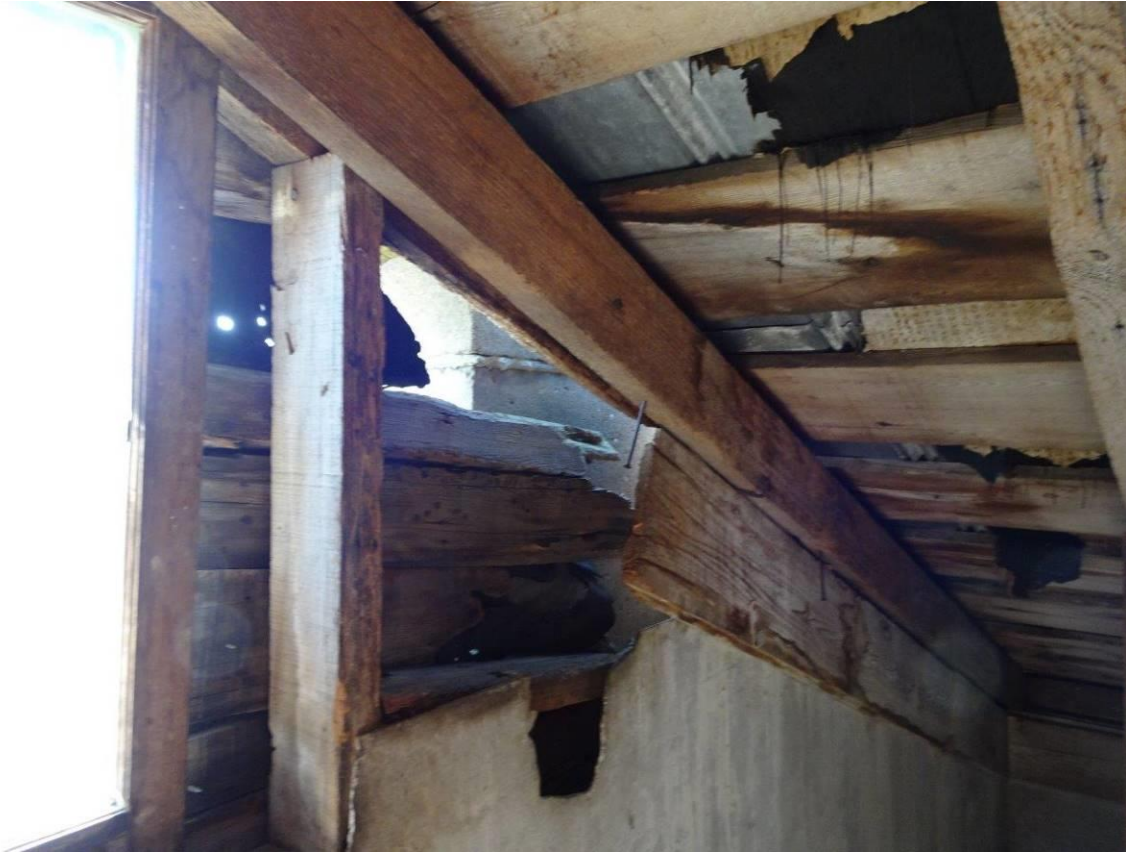
Photo 4.2.17 – Rotted Exterior Wall Sheathing and Interior Wall Sheathing at Attic / Loft
