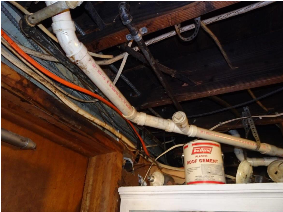
Photo 4.1.31 – Electrical Run Loose – Needs Engineering Review and Repairs
