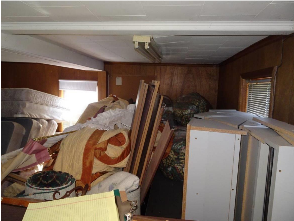
Photo 4.1.30 – Congested Combustible Fire-Hazard Storage Connected to Residential Occupancies
