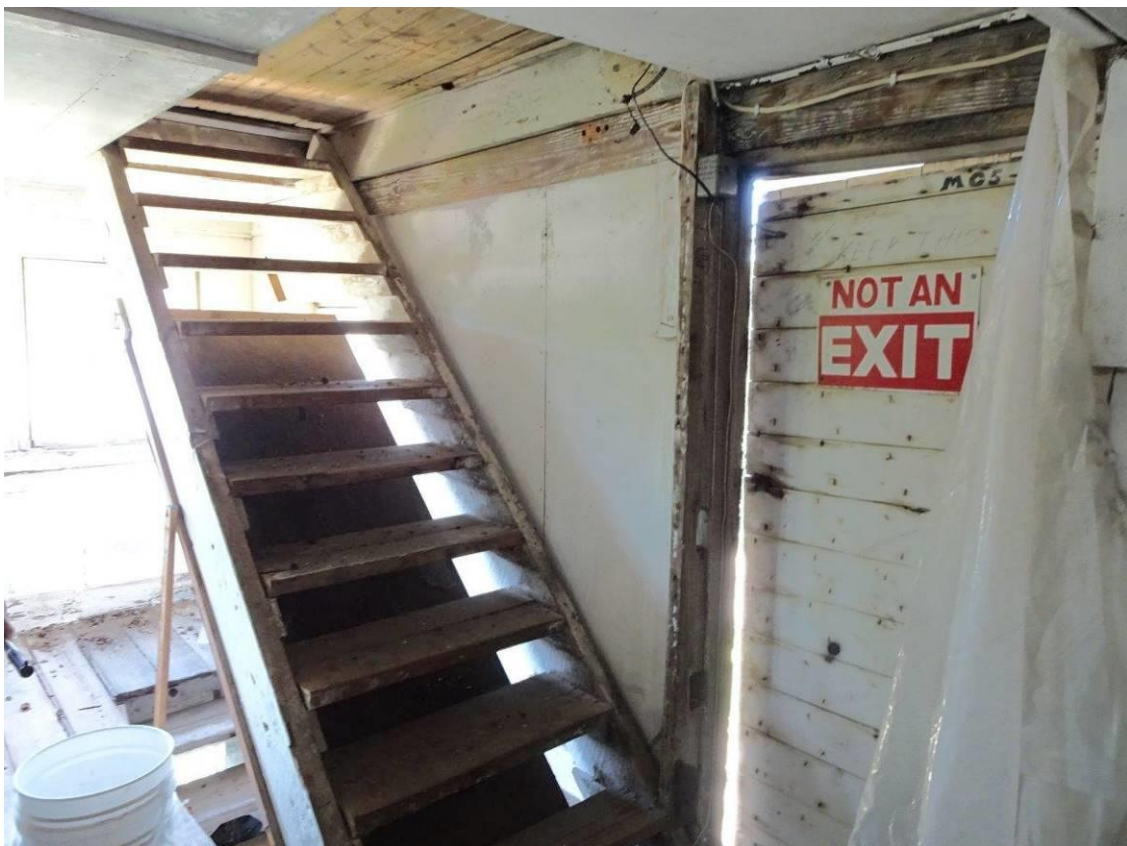
Photo 4.2.24 – Interior Open Stair with No Handrails or Guardrails
