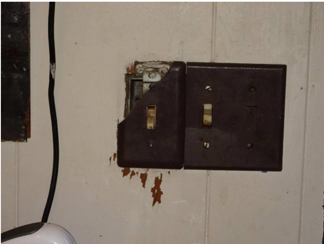
4.1.20 – Broken Receptacle Covers with Exposed Wiring
