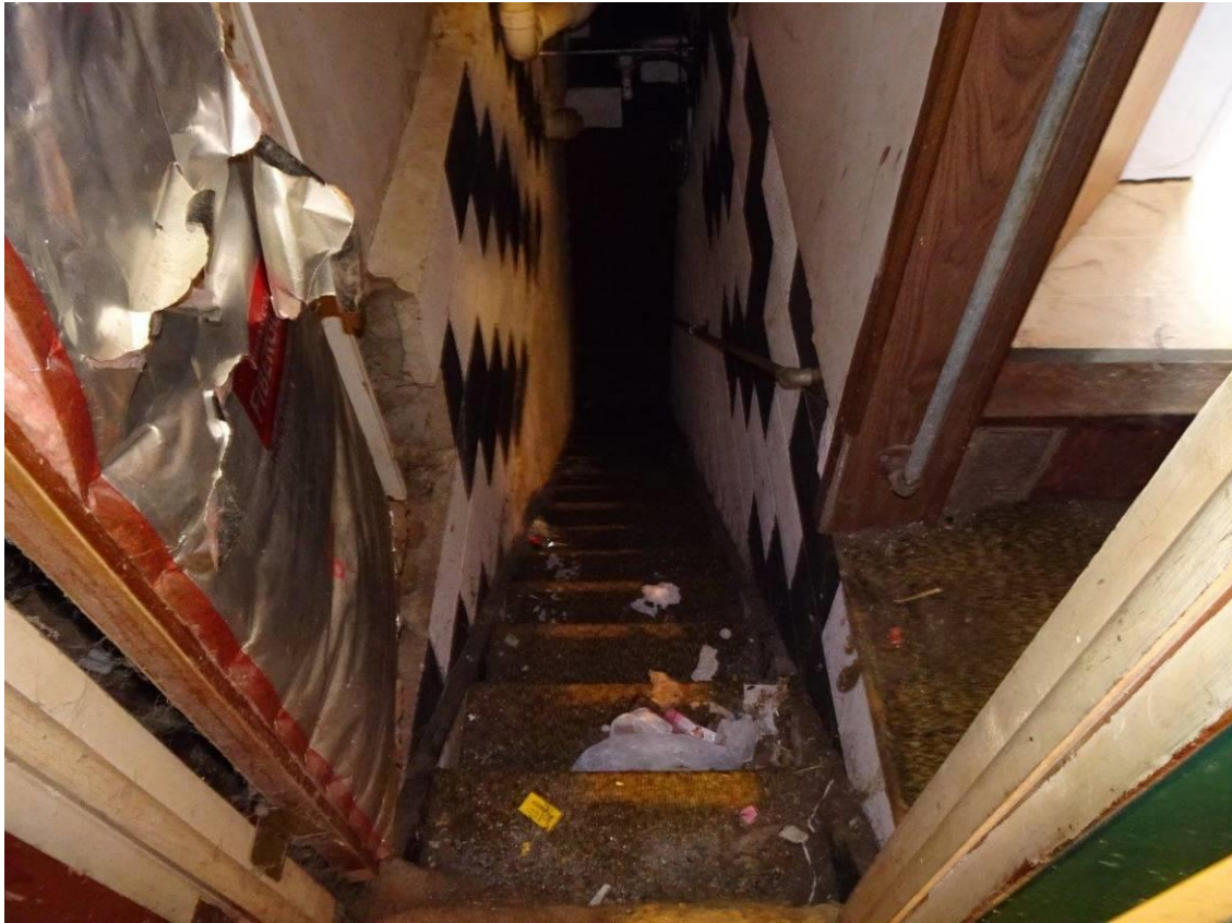
Photo 4.1.7 – Stair to Basement with Step-Down Side Entry to Kitchen and Non-Full Length Handrail
