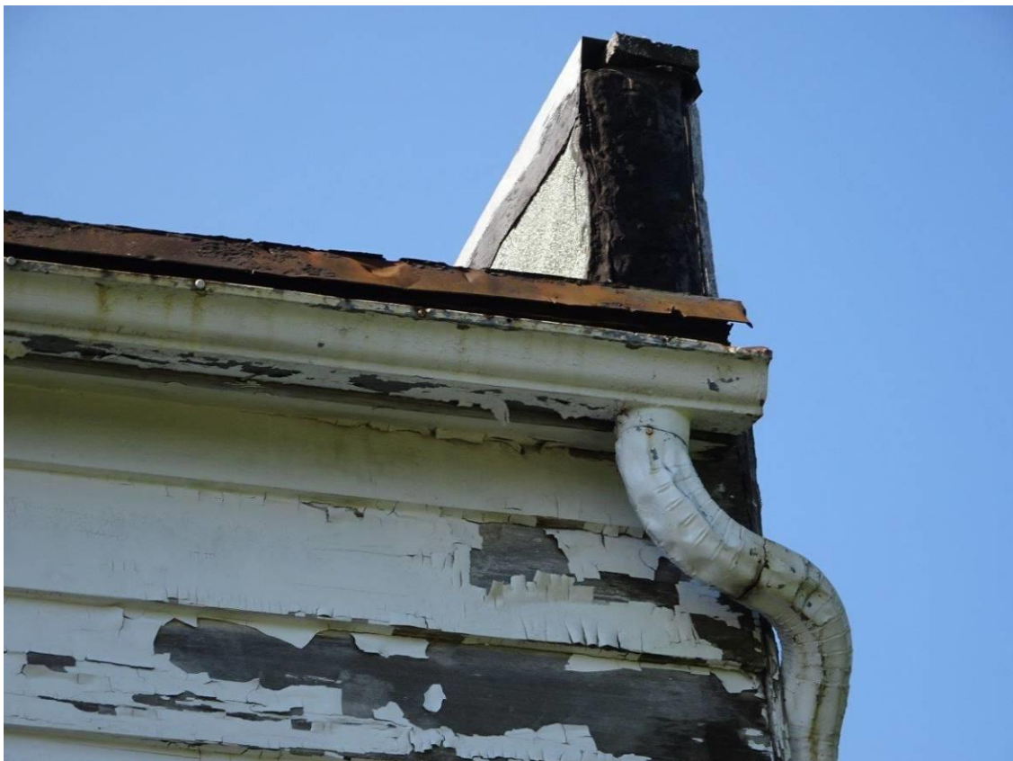
Photo 4.1.14 – Rotting Parapet Walls, Rusting and Failing Roof Edge Flashing and Neglected Paint
