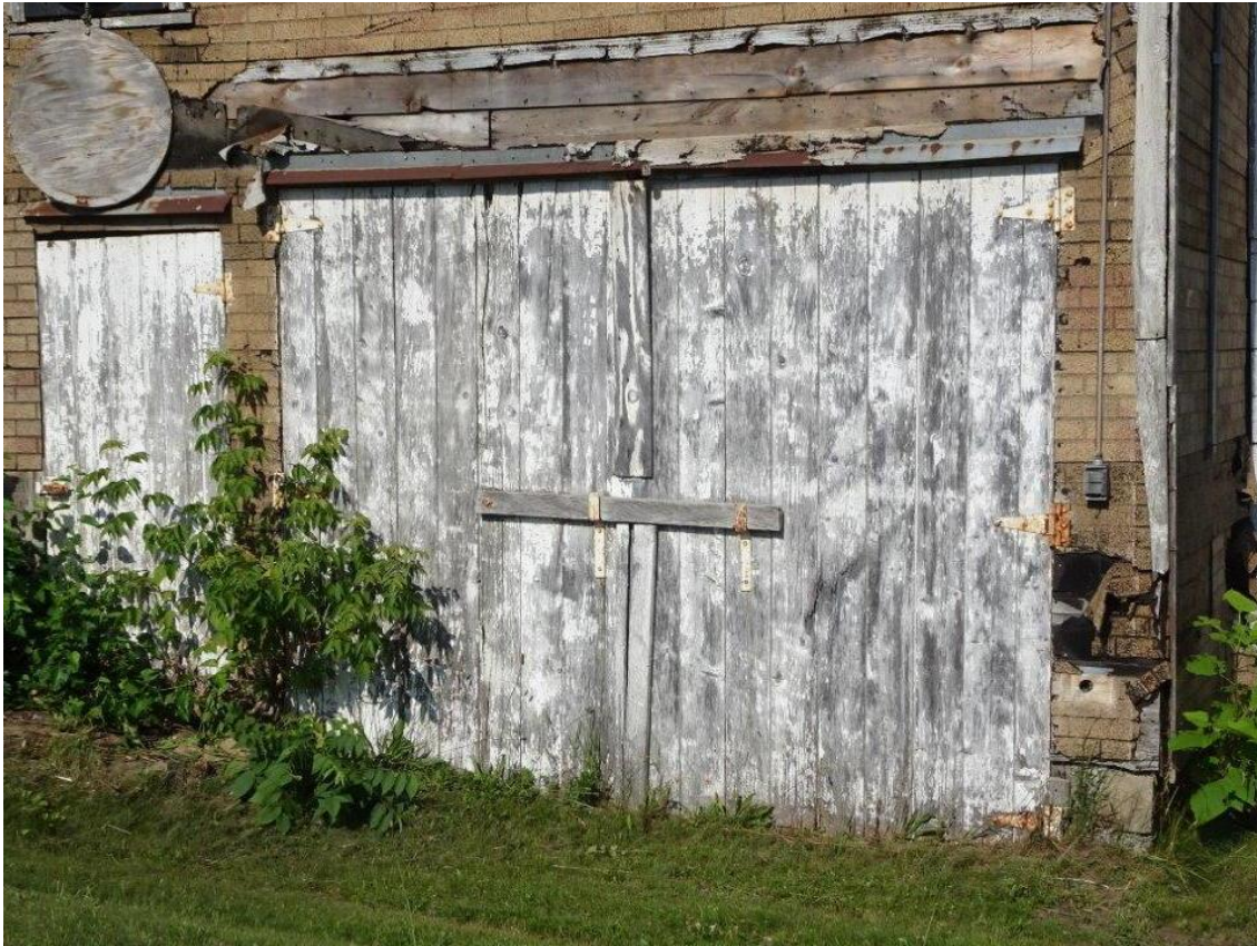
Photo 4.2.27 – Unsecured Exterior Doors with Drop Board and Bracket Access
