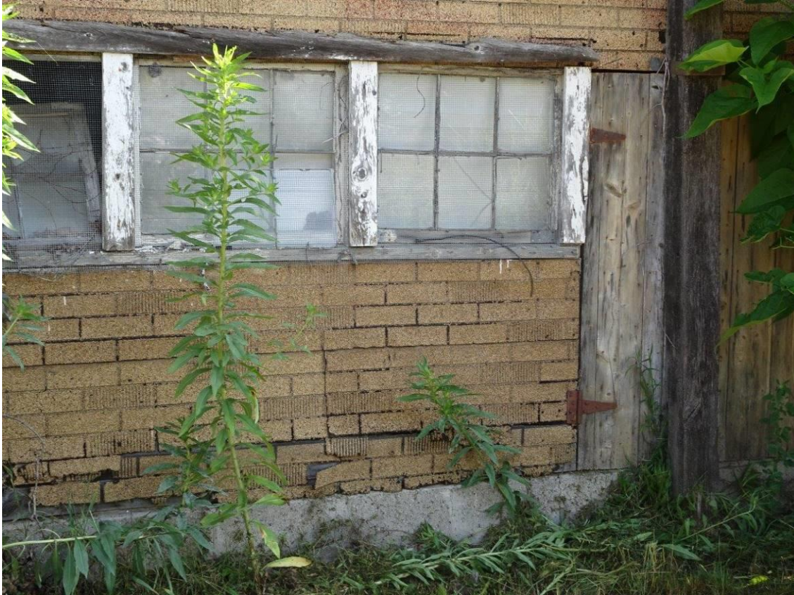
Photo 4.2.11 – Rot at Base of Walls from Water Infiltration
