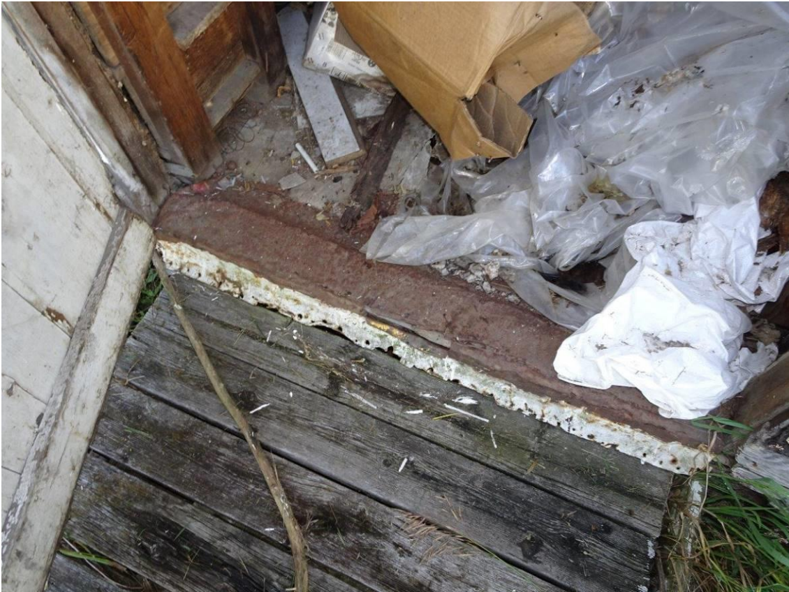
Photo 4.3.6 - Rotting Storage Packed Tight in Building Hindering Full Entry or Floor Structure Review
