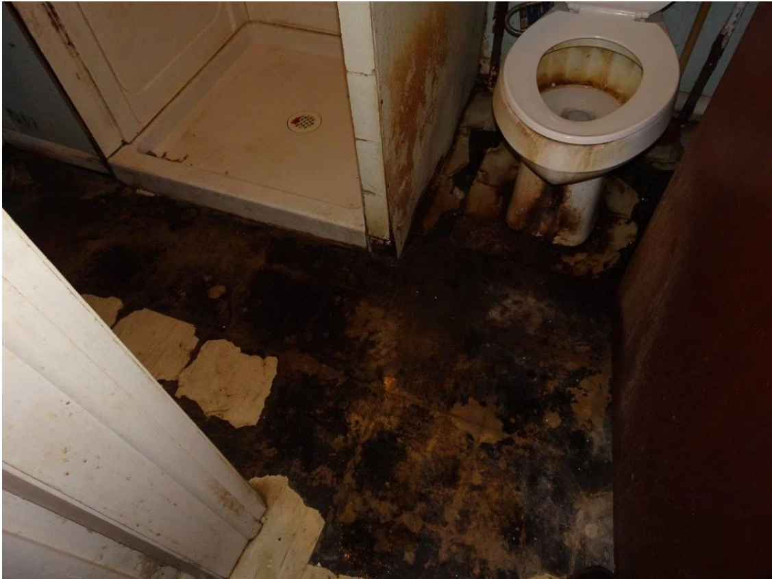
Photo 4.1.21 – Saturated and Rotting Bathroom Floor with Wall Mold
