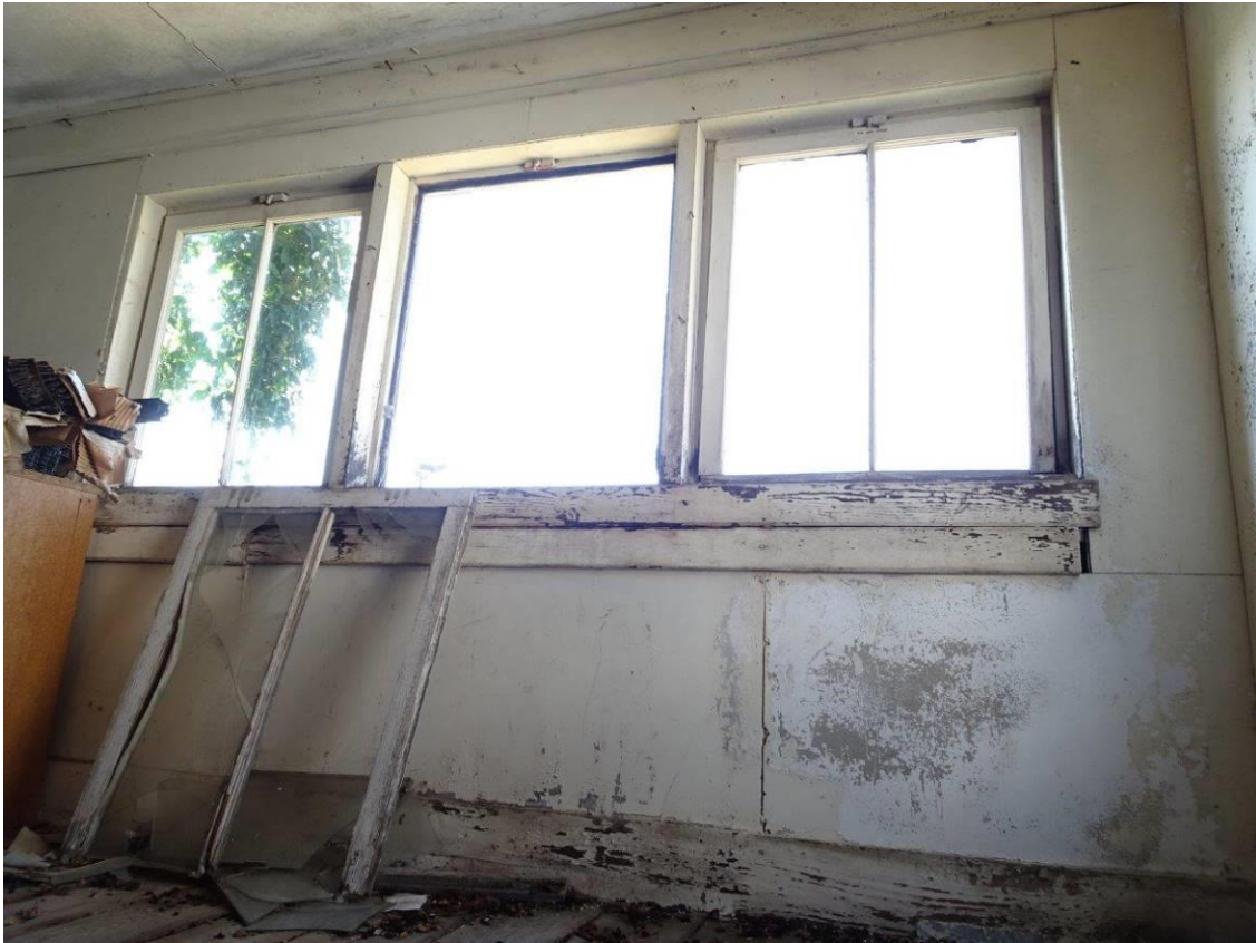
Photo 4.2.7 – Degrading Weathered Interior Walls at Missing Windows
