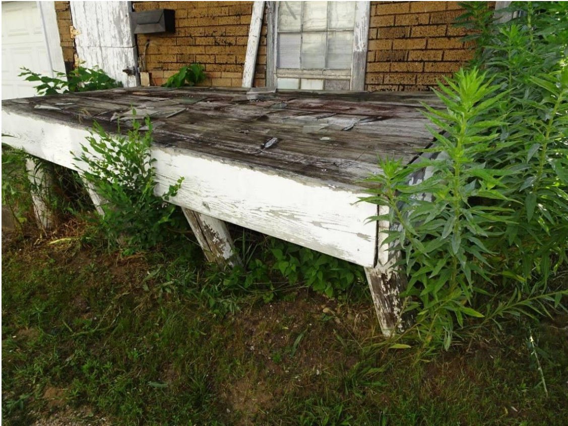
Photo 4.2.23 – Dilapidated Wood Platform Collapsing Away from Building
