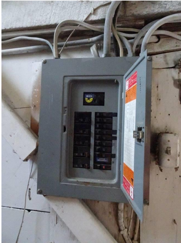
Photo 4.2.21 – Existing Electrical Service Panel and Exposed Wiring
