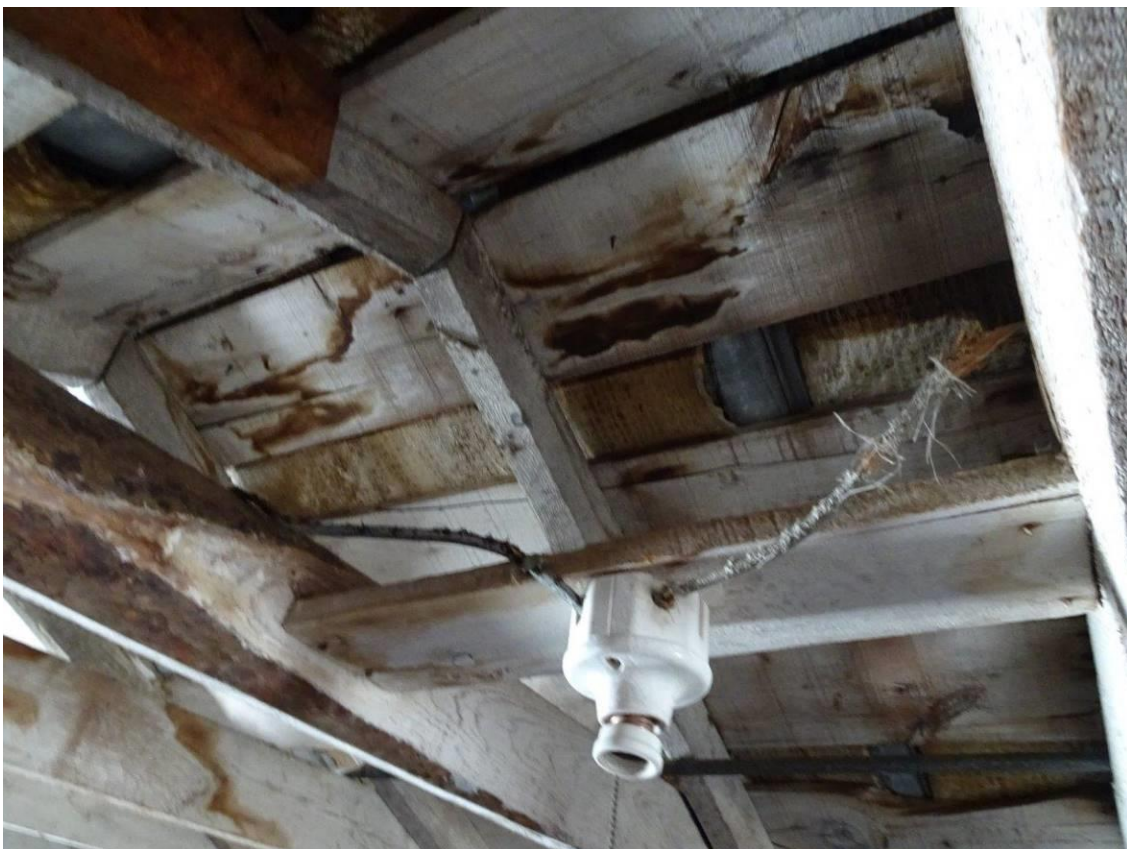
Photo 4.2.30 – Exposed Outdated Wiring with Cracked and Missing Sheathing
